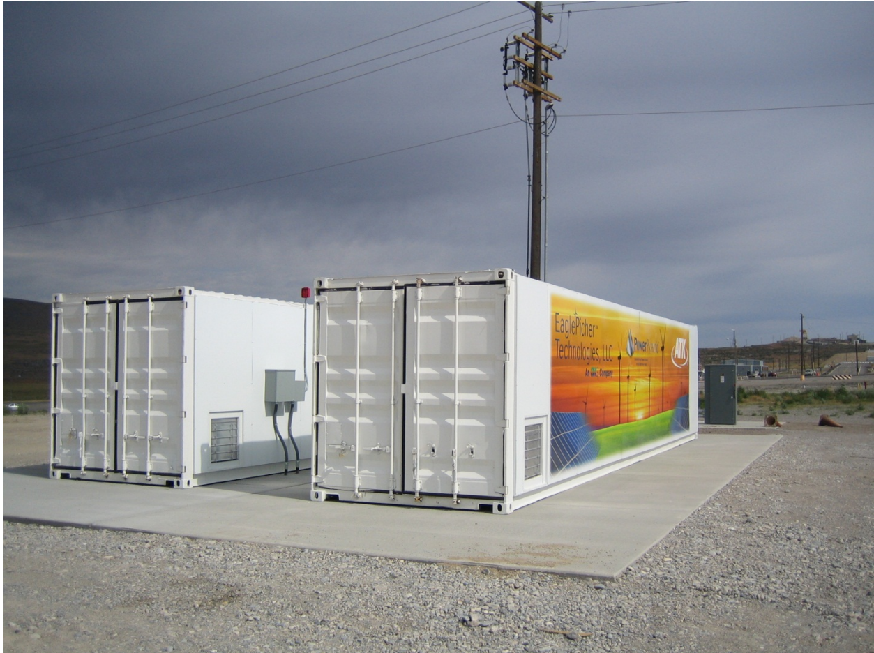
Figure 8 - 300KW Battery Storage System
