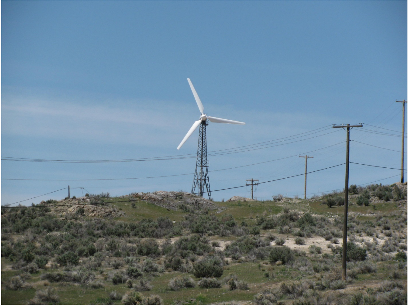
Figure 3 - Wind Generator in Operation
