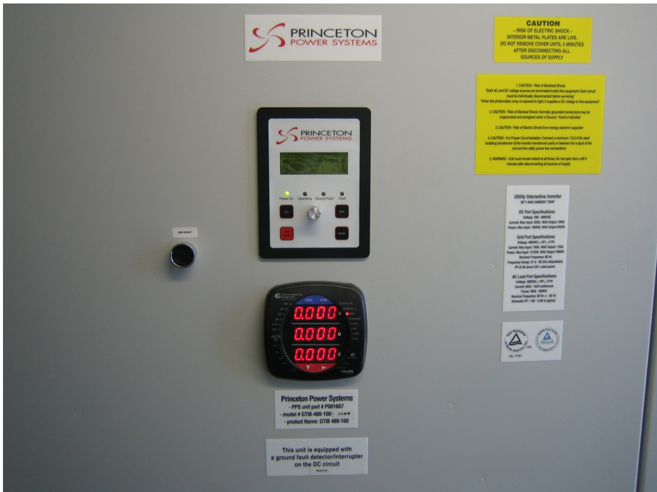
Figure 10 - Battery System Inverter
