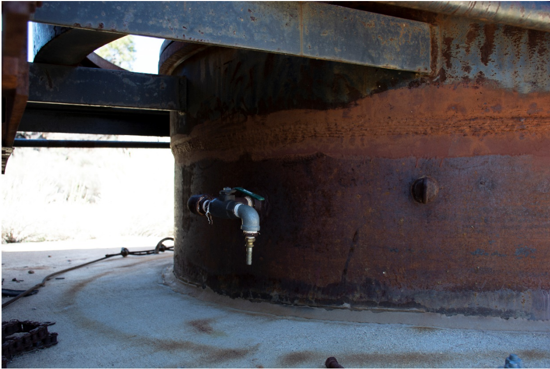
PHOTO NO. 11 CLOSER VIEW OF PETCOCK VALVE ON SOUTH SIDE OF VENT PIPE FACING THE WEST
