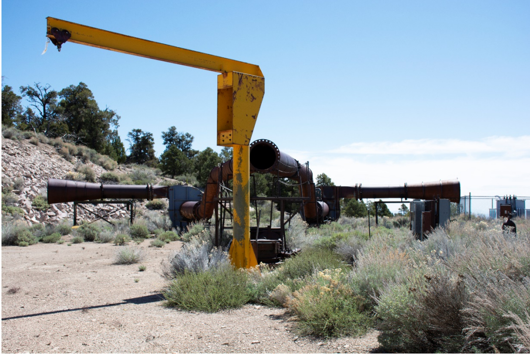
PHOTO NO. 1 GENERAL VIEW OF VENT HOLE SYSTEM WITH CRANE AND BUFFALO BLOWERS IN BACKGROUND FACING THE EAST
