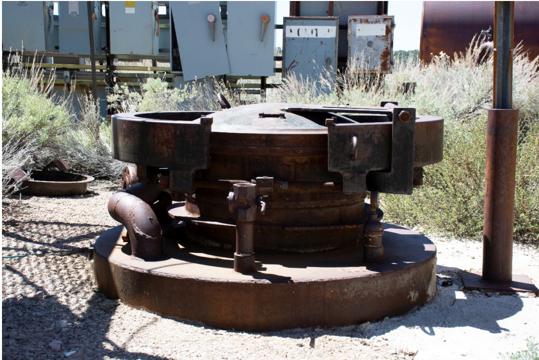
PHOTO NO. 7 CLOSER VIEW OF TUBE TURN CONTAINMENT DOOR, YOKE STYLE CLAMP CLOSING MECHANISM, AND VENT PIPE FACING THE SOUTH
