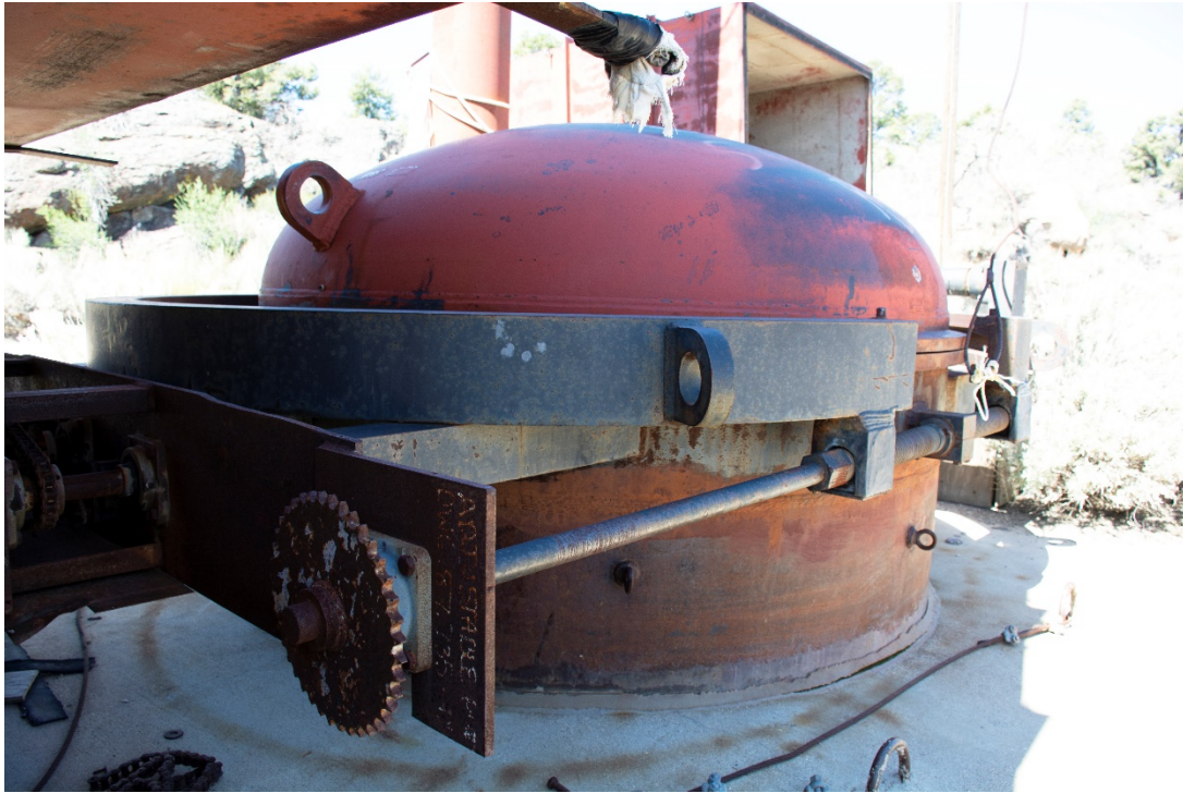
PHOTO NO. 12 CLOSER VIEW OF YOKE STYLE CLAMP CLOSURE MECHANISM FACING THE NORTHWEST
