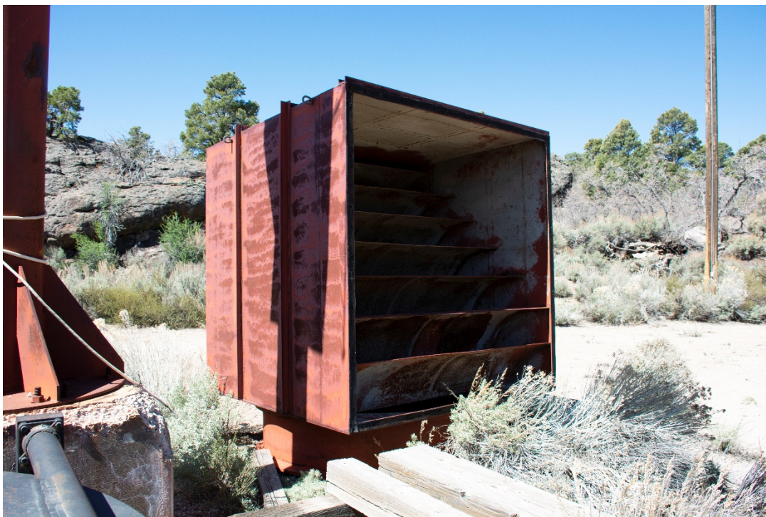
PHOTO NO. 16 CLOSER VIEW OF CONDUIT ELBOW WITH LOUVERED DUCTING FACING THE SOUTHWEST
