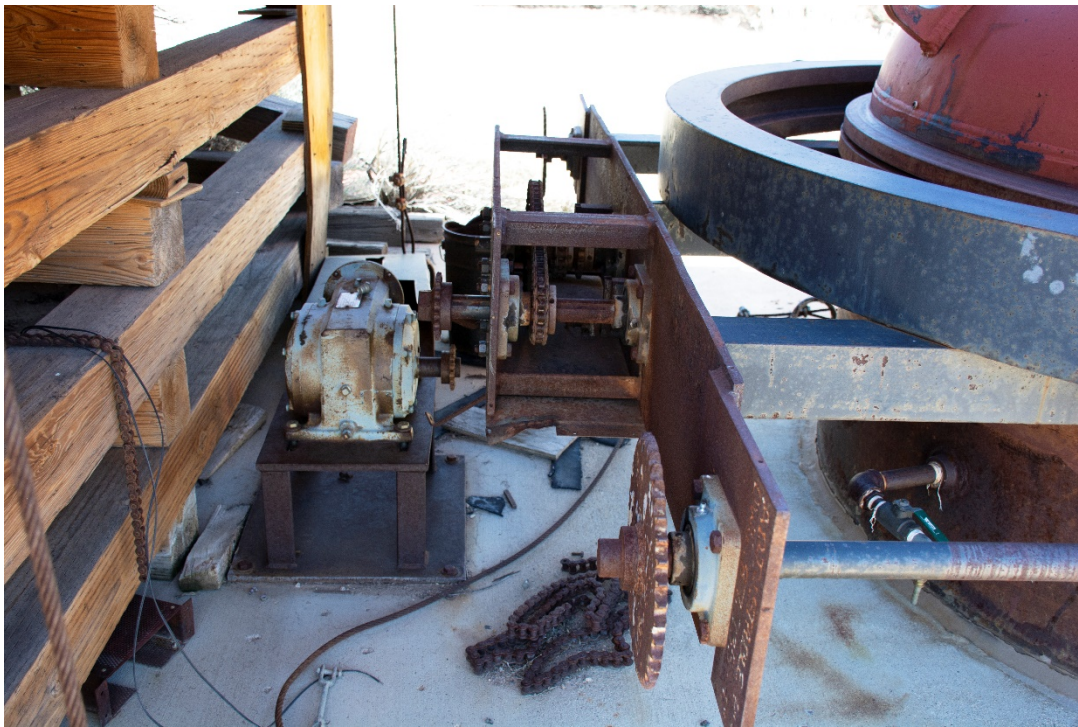
PHOTO NO. 10 CLOSER VIEW OF ELECTRIC MASTER XL SPEED REDUCER GEAR BOX, GEARS, AND THREADED OPERATING BOLTS OF YOKE STYLE CLOSURE MECHANISM FACING THE SOUTHWEST
