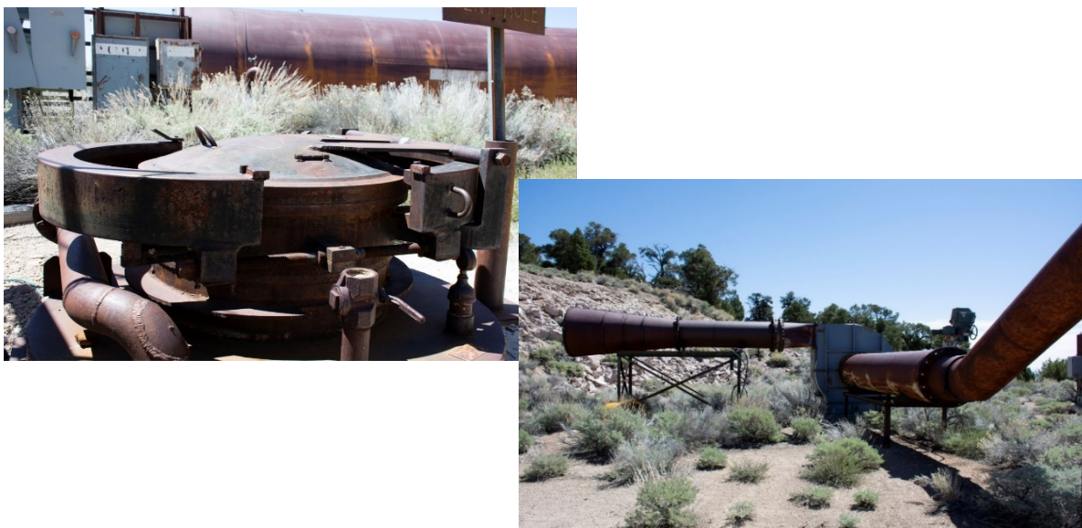
Figure 2. (Top left) detail of yoke-style closure mechanism with grooved interiors that close around rims on the vent casing and the turn-tube containment door, facing southwest (Photo: DSC_5161, DRI 2020); (bottom right) detail of northern vent line, remote-controlled damper section, and Buffalo Blower, facing east (DSC_5122, DRI 2020).
