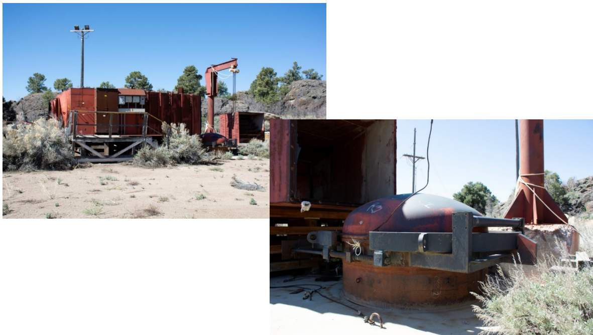
Figure 3. (Top left) overview of U12n Vent Hole #2 showing, from left to right, the vent conduit, containment door, crane, and conduit elbow (Photo: DSC_5069, DRI 2020); (bottom right) tube-turn containment door and yoke-style clamp mechanism in position over the vent pipe casing (Photo: DSC_5107, DRI 2020).
