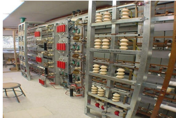
Capacitor Bank Units
