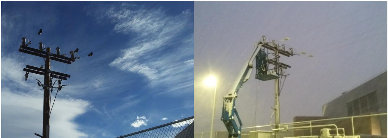
Figure 2. Tier 0 laboratory prototypes being tested at the medium voltage outdoor test area (MVOTA) at NREL in Golden CO. The weather during our tests was quite variable, changing from sunny and warm to heavy snow in 24 hours.
