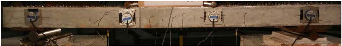
(a) flexure cracks at Total Load of 15-kips
