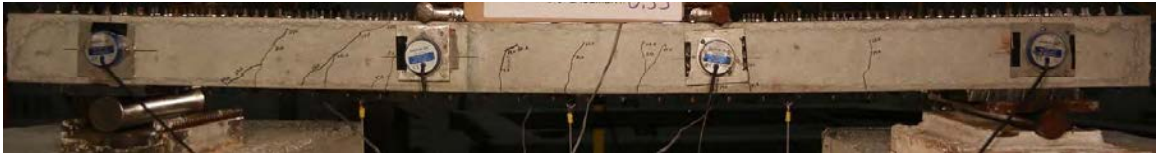
(b) Shear Cracks at Total Load of 20-kips
