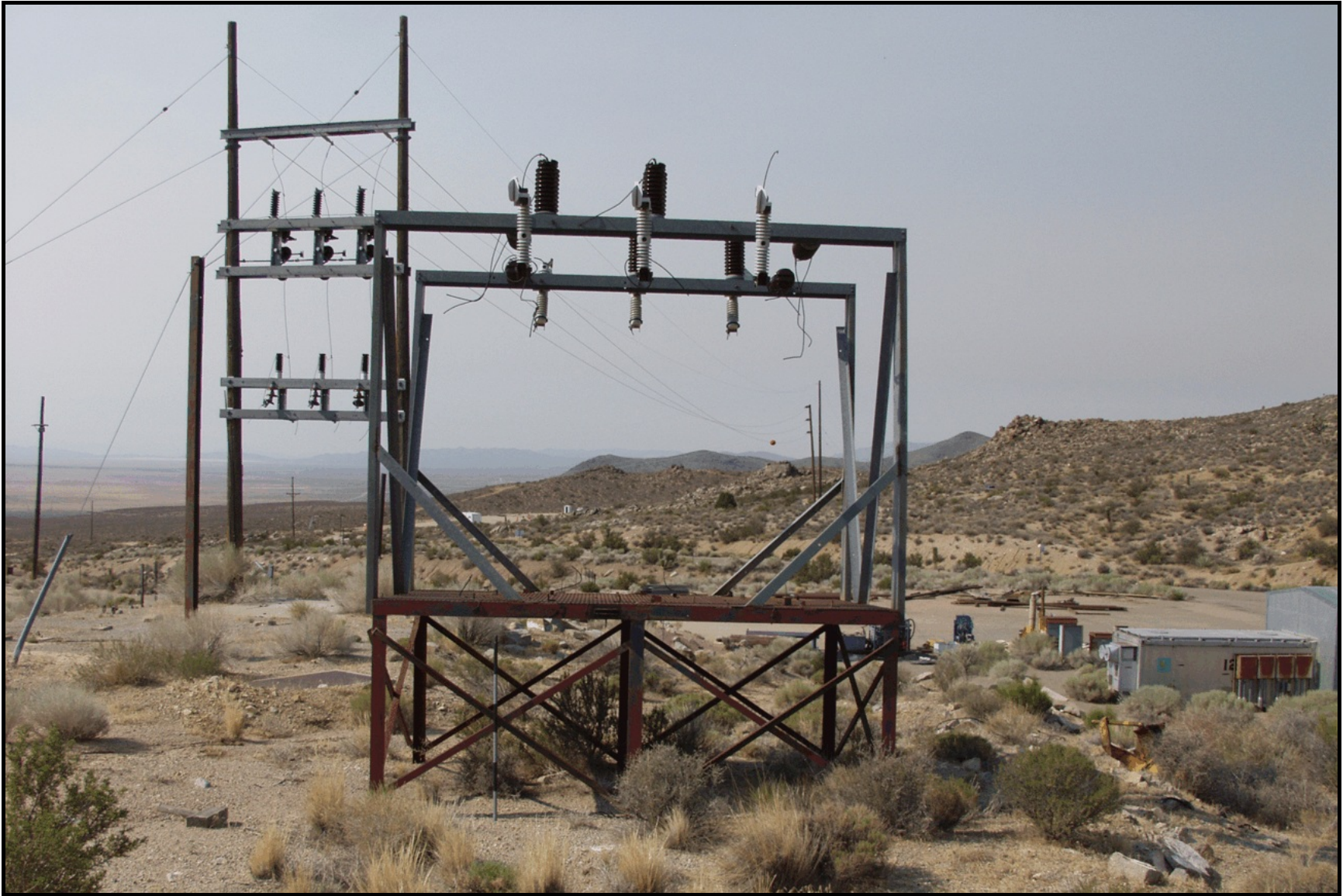
Figure 137. Structure 4, electric substation, view south (2013).
