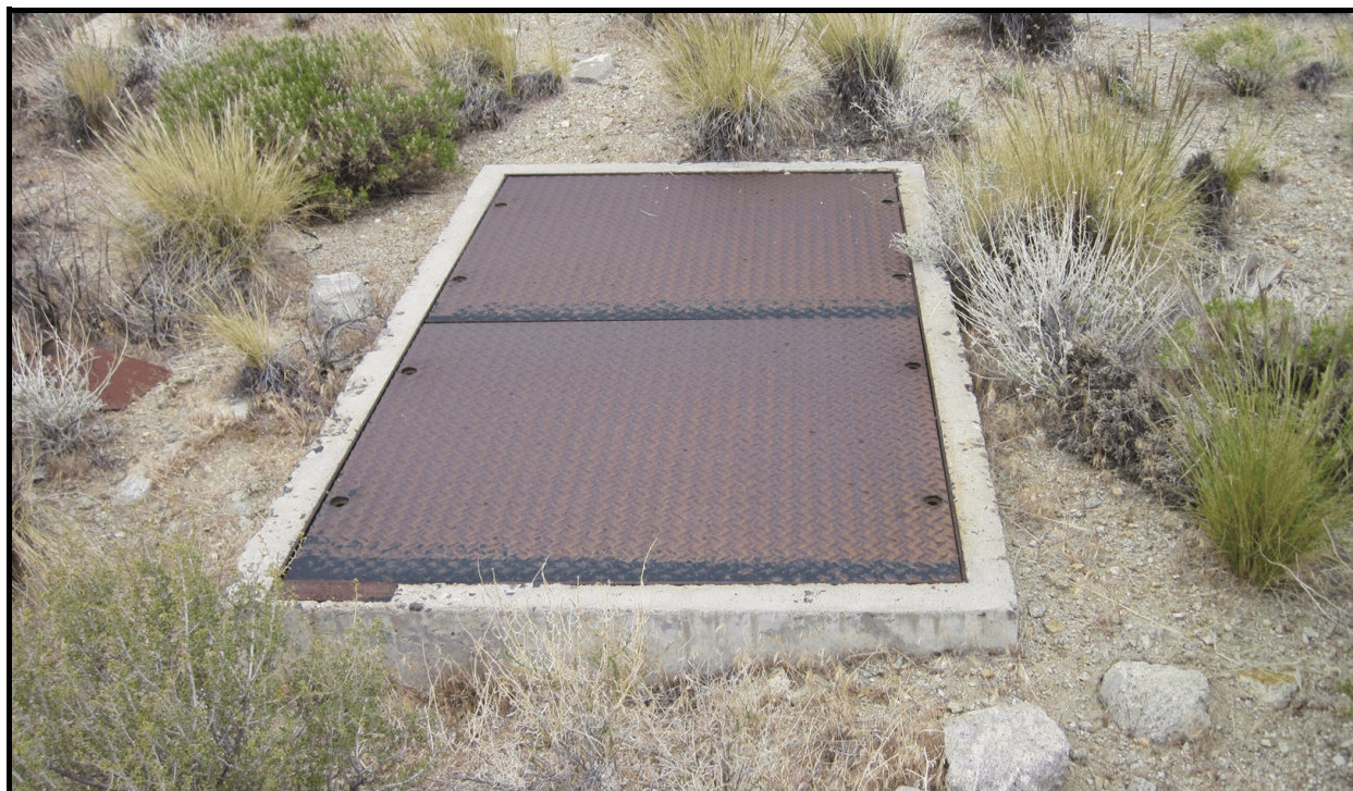
Figure 192. Feature 40, electric cable vault, view northwest (2013).
