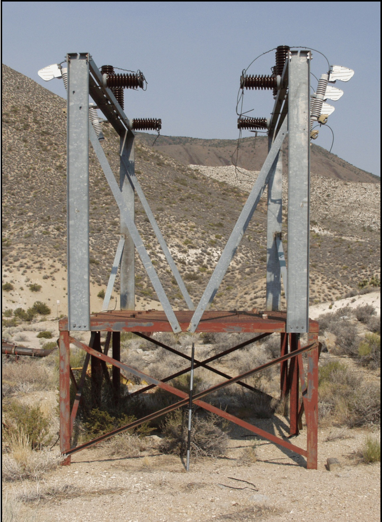
Figure 138. Structure 4, electric substation, view west (2013).
