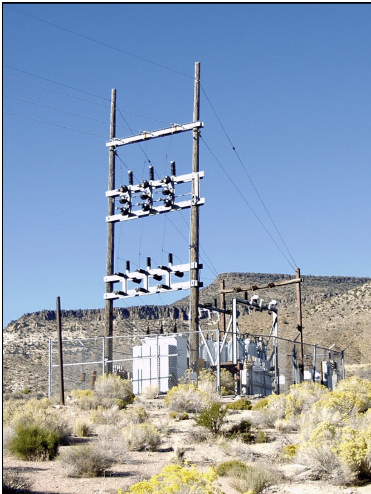
Figure 202. Feature 47, main electric substation, view northwest (photograph on file).
