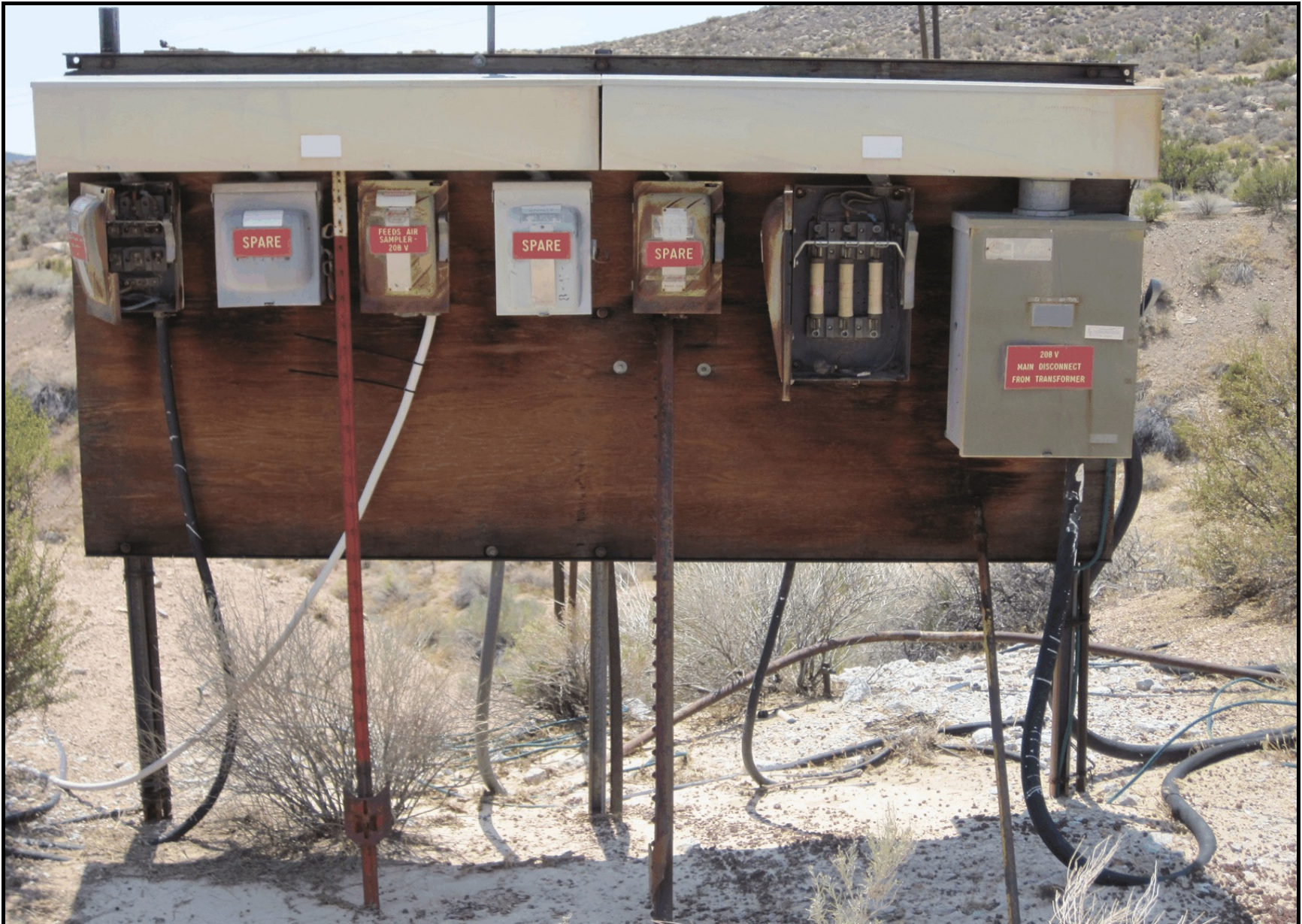
Figure 198. Feature 46, electric panel, east side, view southwest (2013).
