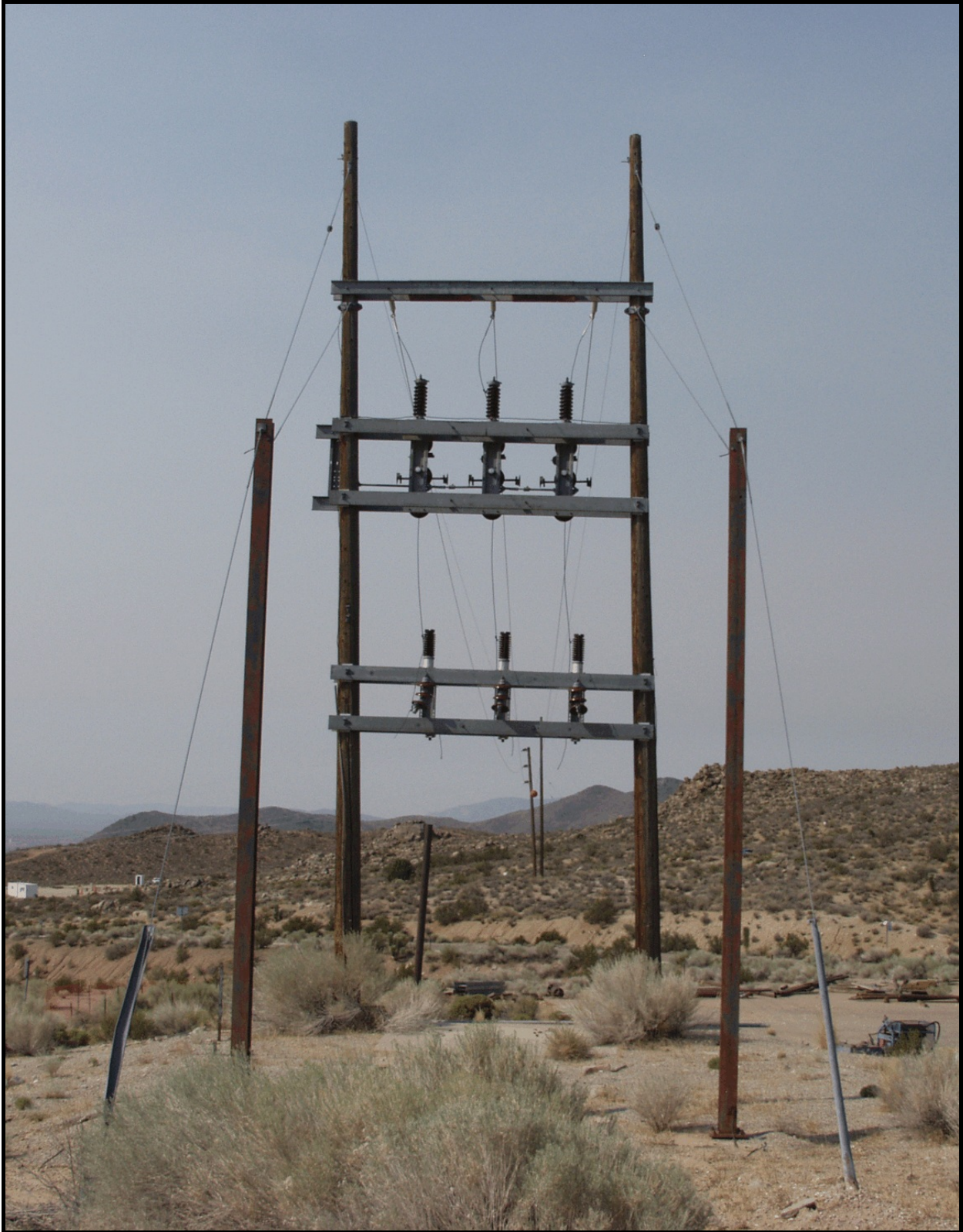
Figure 201. Feature 47, main electric substation, view southwest (2013).
