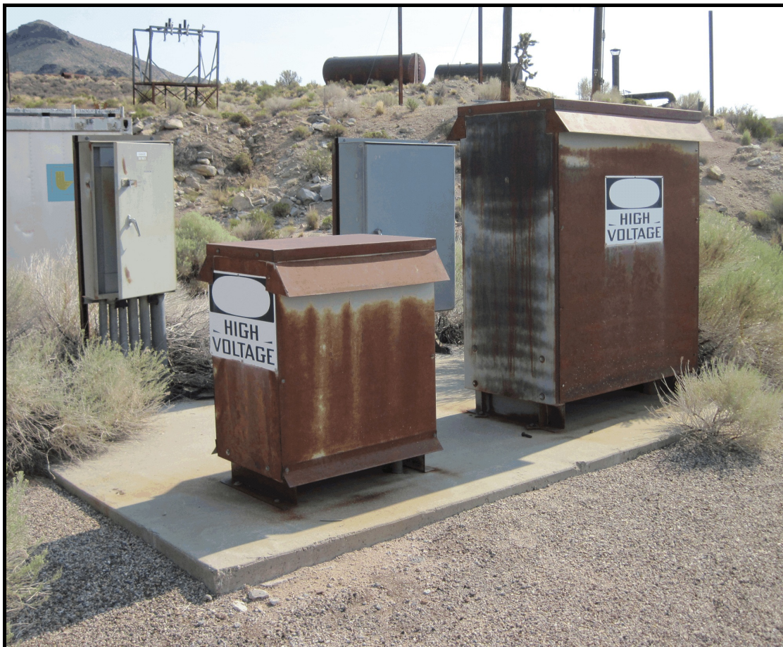
Figure 197. Feature 45, electrical equipment, view northeast (2013).
