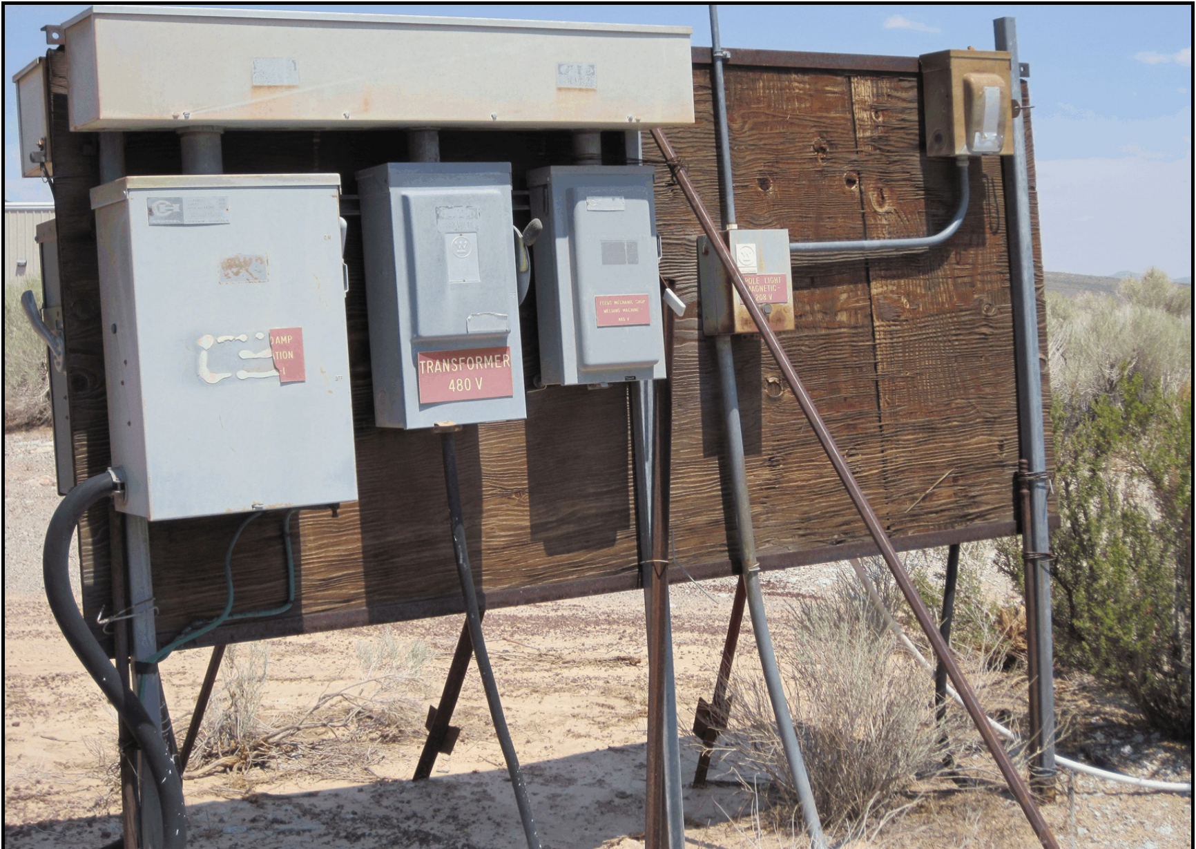
Figure 199. Feature 46, electric panel, west side, view east (2013).
