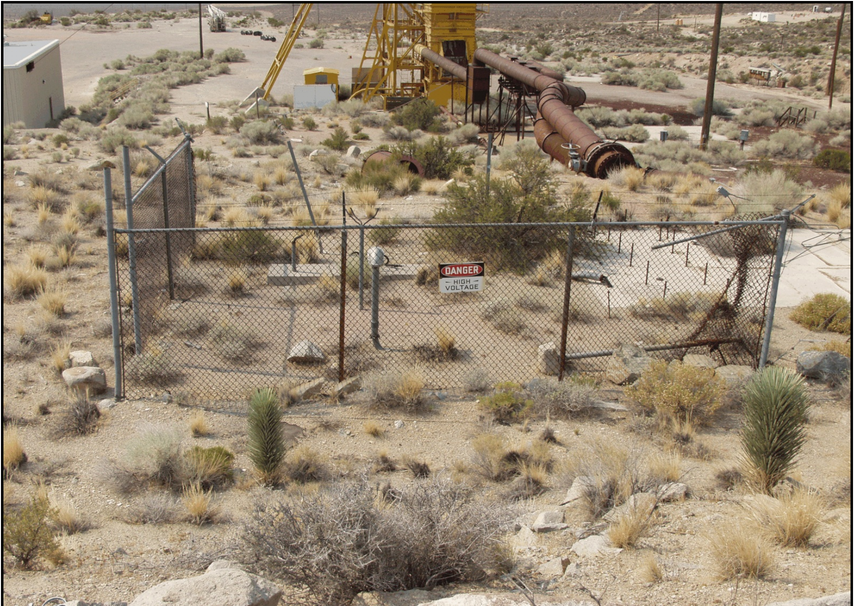
Figure 203. Feature 48, electric substation, view south (2013).
