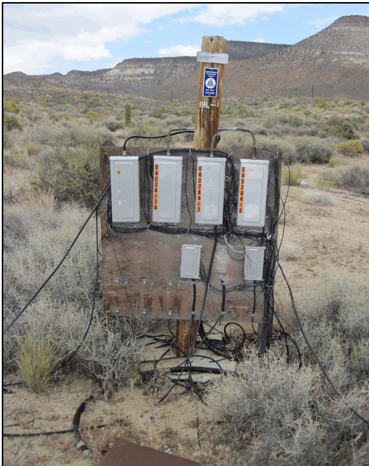
Figure 195. Feature 43, telephone panel, view north (2013).
