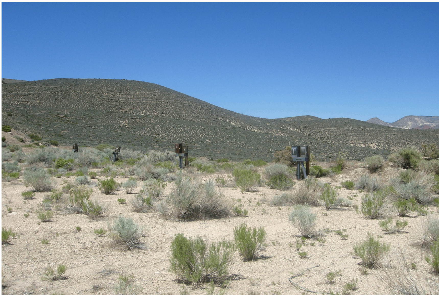
Figure 57. U16a Tunnel Feature 15, switch boxes, view northwest (2011).
