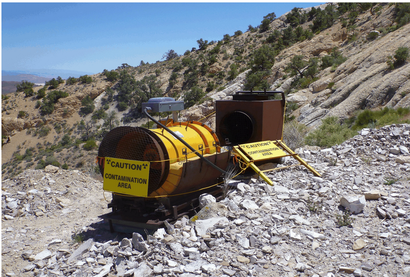
Figure 99. U16a Tunnel Feature 42, U16a #1 vent and blower assembly, view east (2011).
