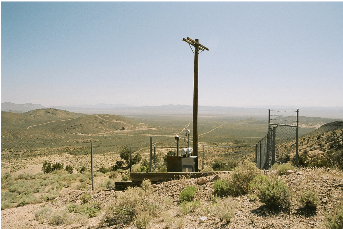
Figure 75. U16a Tunnel Feature 32, plan map and photograph of electrical substation, view east (2011).
