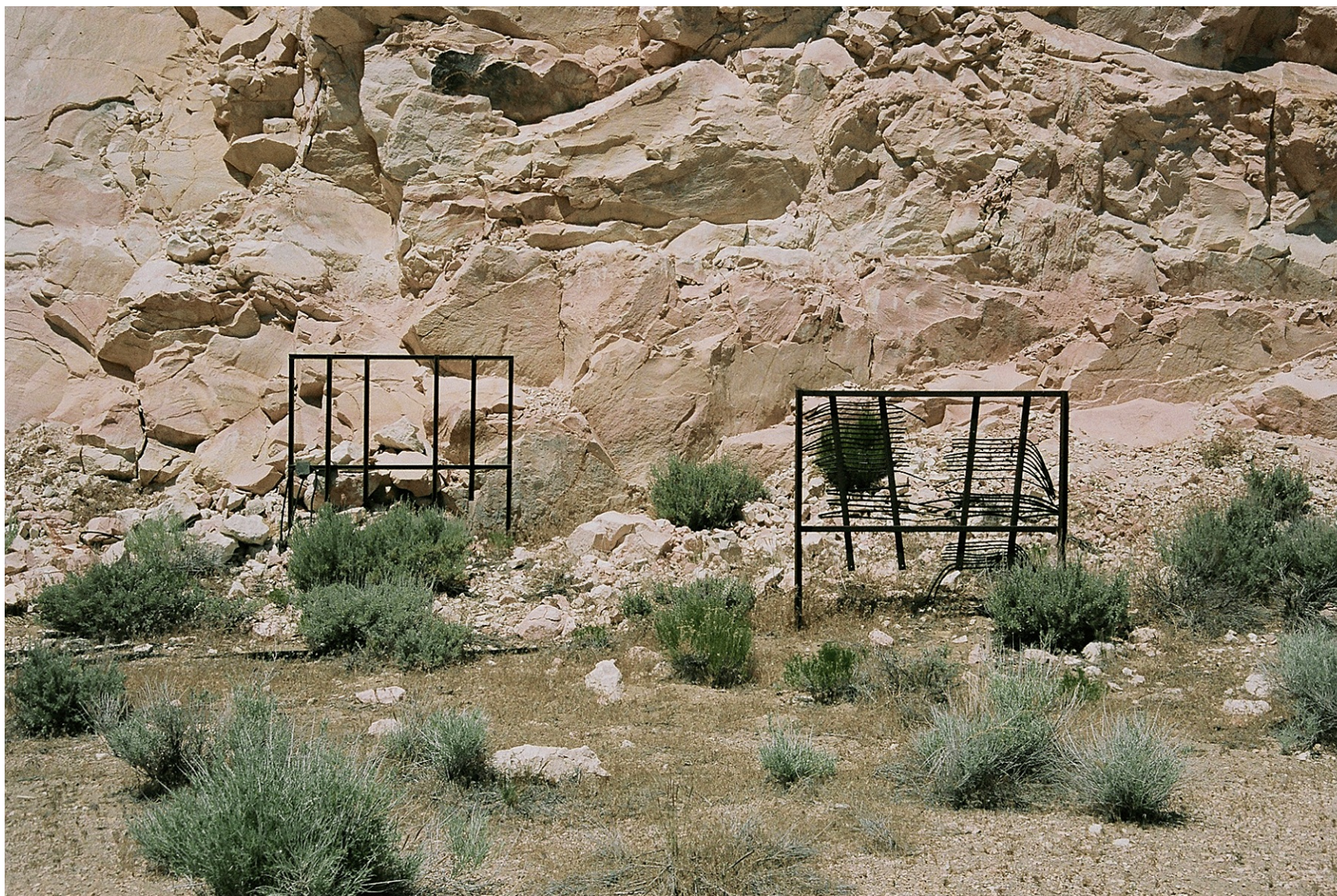
Figure 64. U16a Tunnel Feature 21, electrical panel backboards, view west (2011).
