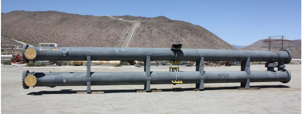
Figure 22 Shell and Tube Heat Exchanger at Site
