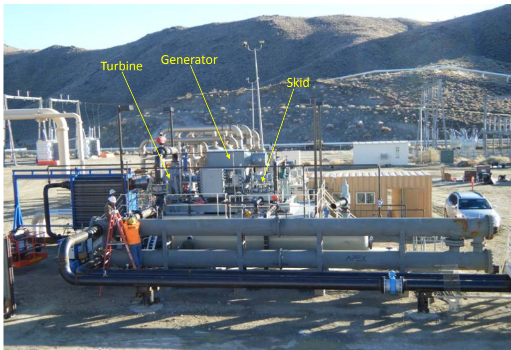
Figure 33 Side View of Completed 1 MW Plant at Coso Geothermal Resource
