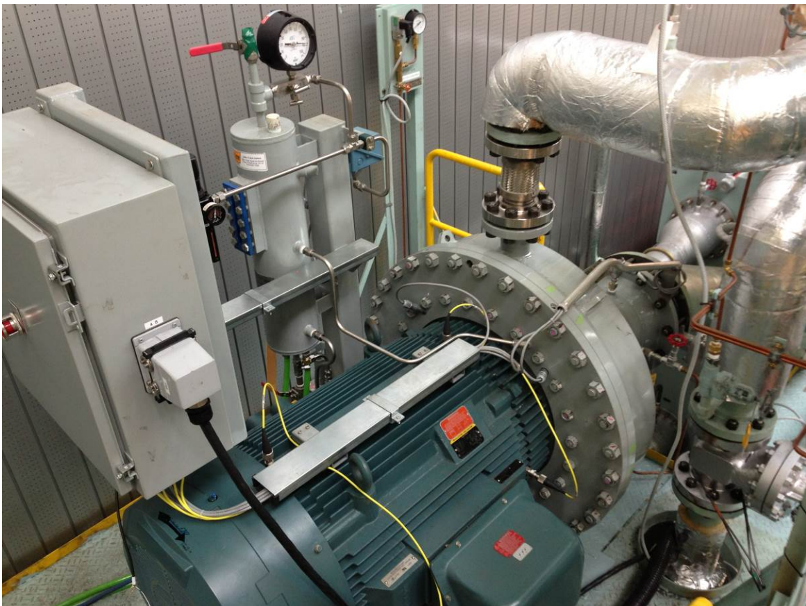
Figure 40 Variable Phase Turbine Operating in Waste Heat Recovery System
