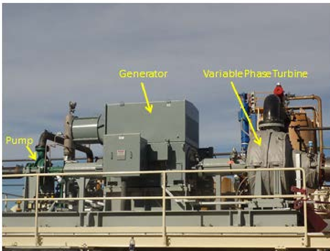
Figure 35 Variable Phase Turbine Power Train during Operation
