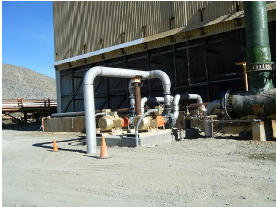
Figure 26 Cooling Water Pumps and Cooling Water Line
