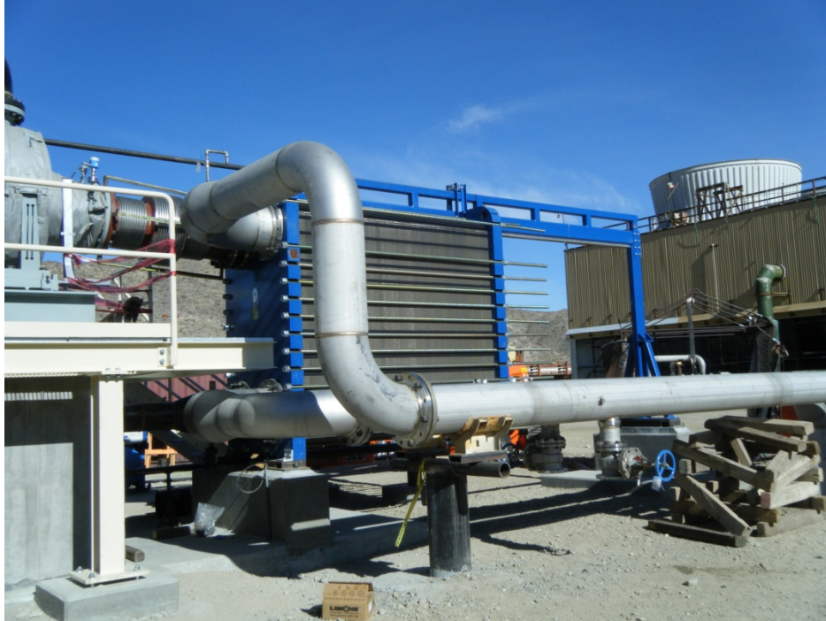
Figure 27 Cooling Water Lines and Condenser
