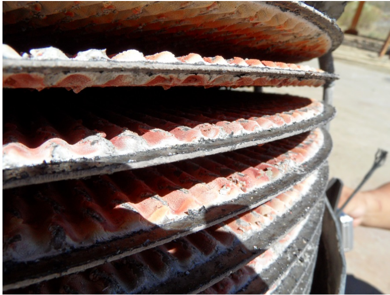
Figure 11 Plate – Fin Heat Exchanger Deposits
