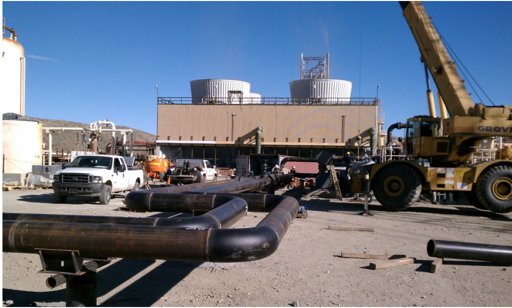
Figure 29 Brine Lines Leading to Heat Exchanger
