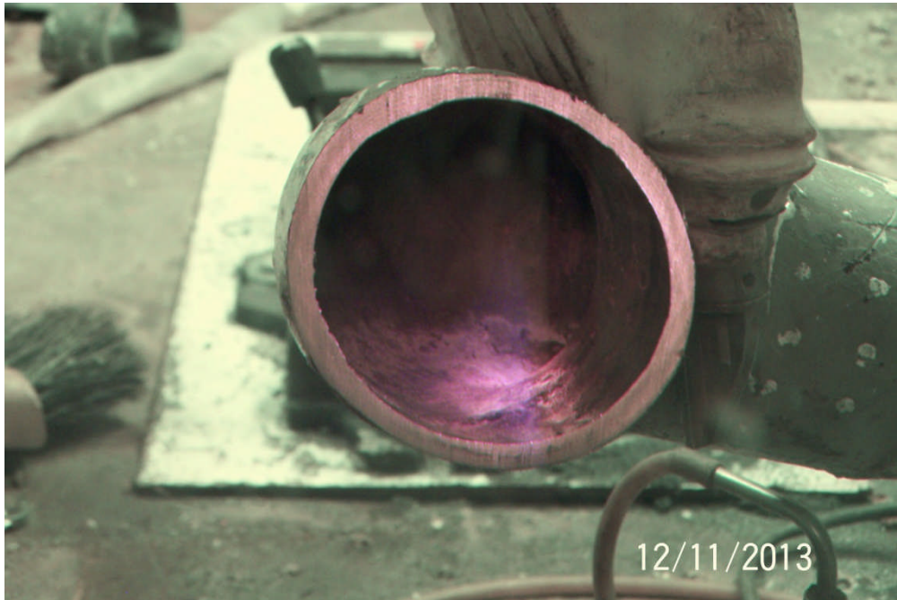
Figure 2-9. Photo of the Inner Wall of the First Elbow of Jumper B – 2.
