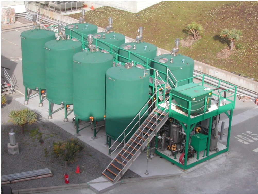
Figure 3: Brown Grease Recovery Demonstration Facility
