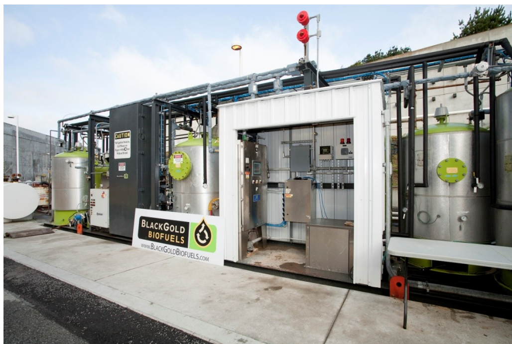
Figure 8: Photo of Biodiesel Conversion Facility
