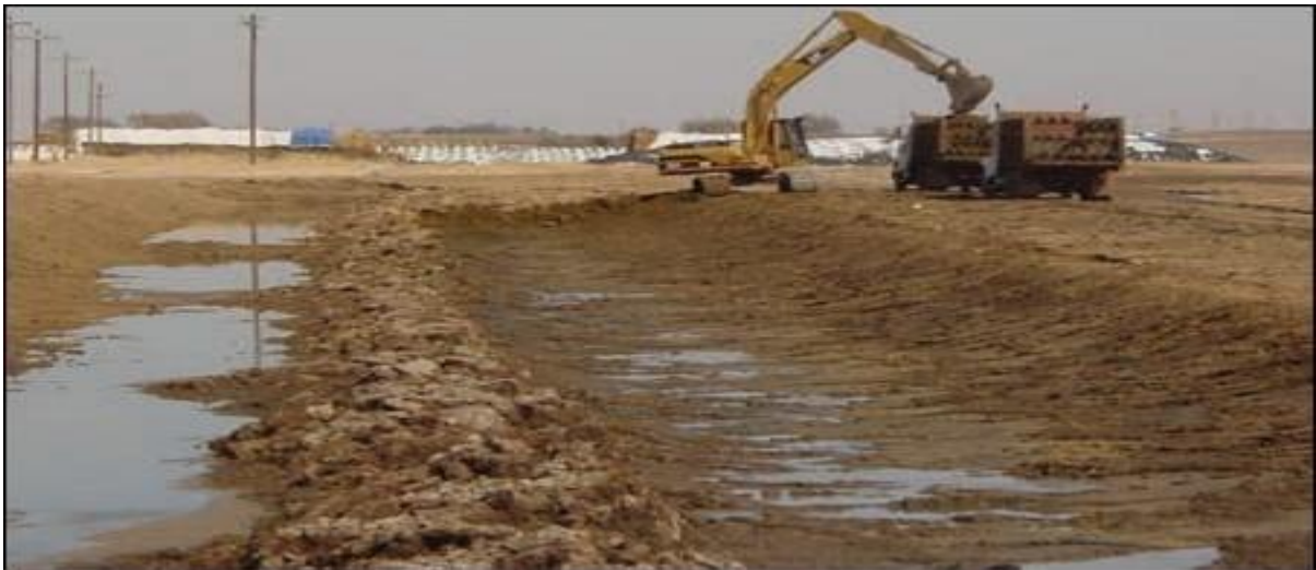
(Figure 3. Gravitational solids separation basin during clean out. The liquid enters the basin in the foreground and slows to allow solids to separate from the water, which continues to flow through the basin and to the lagoon.)
