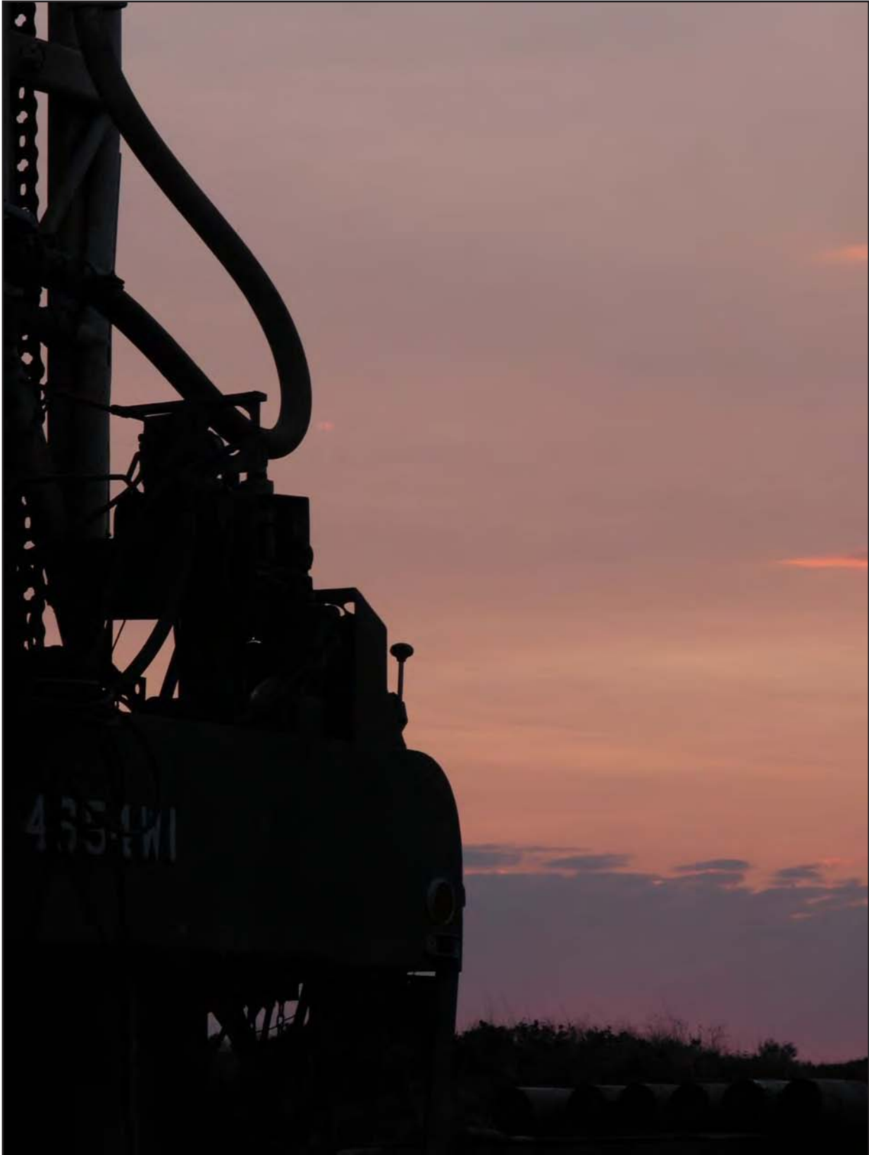
Rig #15 in pre-dawn, June 23, 2006, at SNL-18 drillpad. Photo by Dennis W. Powers.
