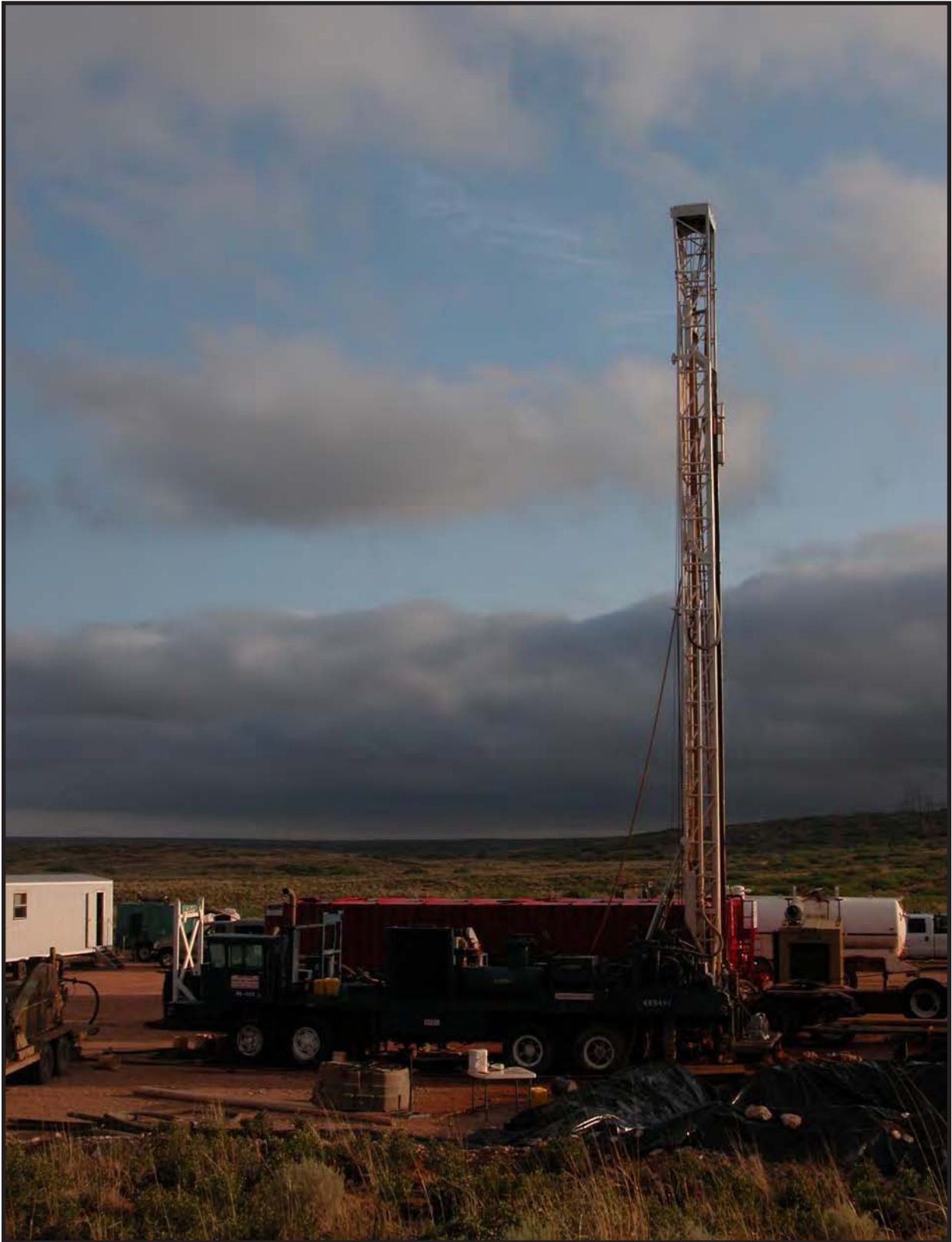
West Texas Water Well Service Rig #15 at SNL-18 on June 23, 2006. Toward north, with the Nash Draw escarpment in the background on the right. Photo by Dennis W. Powers.
