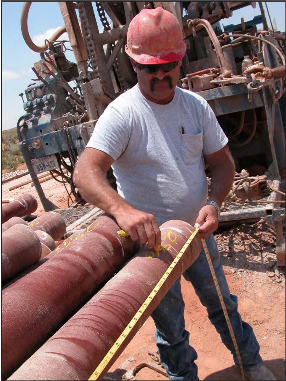
Ronnie Keith (WTWWS) measuring and marking each fiberglass-reinforced plastic casing for SNL-18 prior to installing at SNL-18 on June 29, 2006. Photo by Dennis W. Powers.
