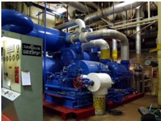
Fig 3a. Pixel image of boiler room
