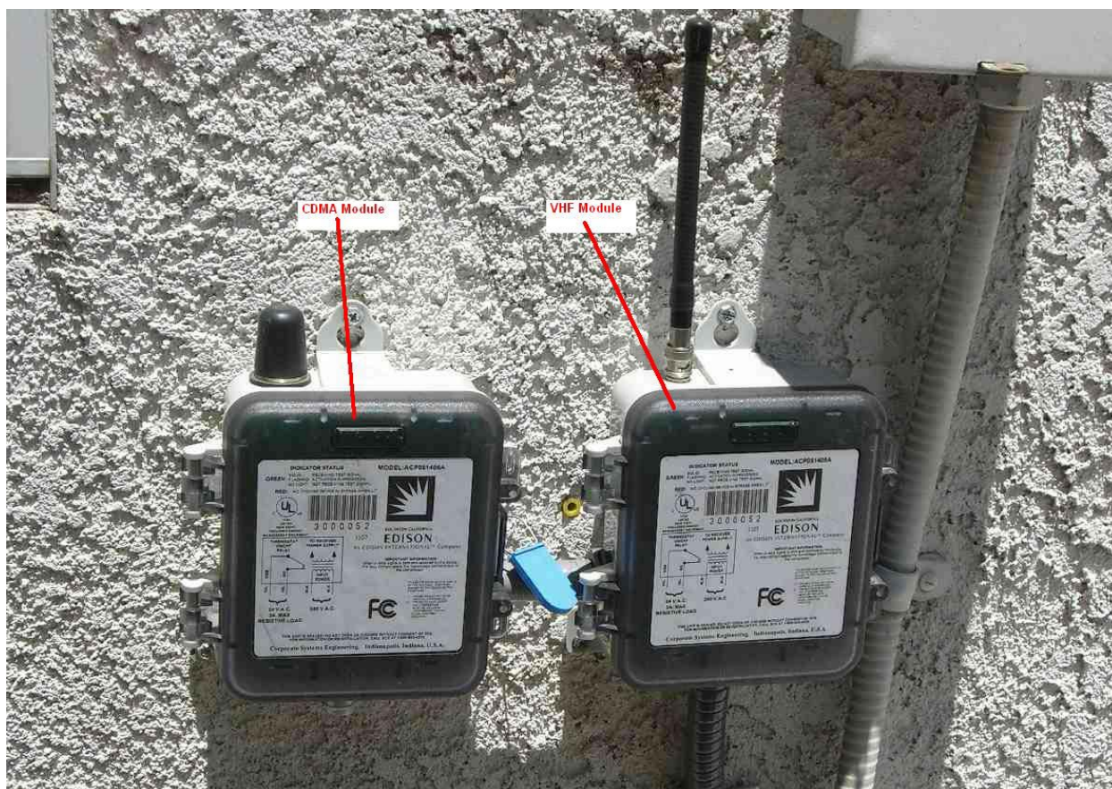
Figure 3.4 SCE AC Load Control Switch
