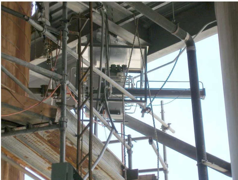
Figure 38. Receiver unit mounted on the Wabash River gasifier
