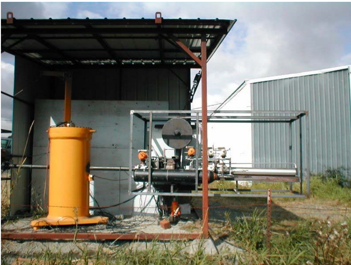
Figure 28. Field prototype “auto-GAP 1” sensor mounted on the EGS1 pressure vessel
