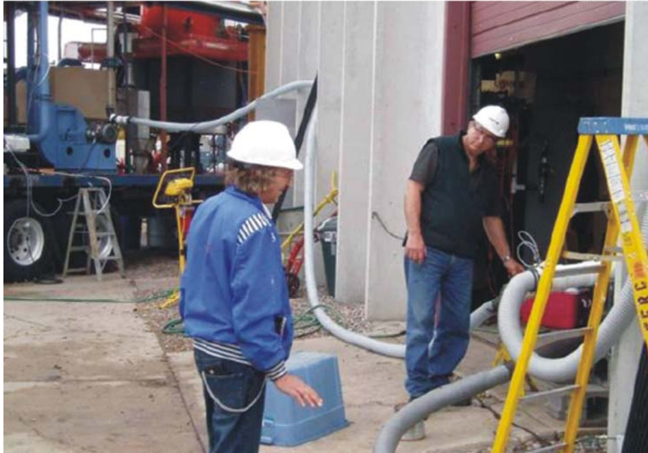
Figure 11. Gas piping from gasifier trailer to engine located in the building.
