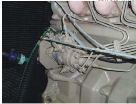
Figure 13. Diesel fuel pump and governor.
