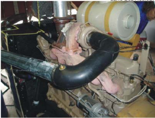
Figure 12. Gas piping to turbo intake.
