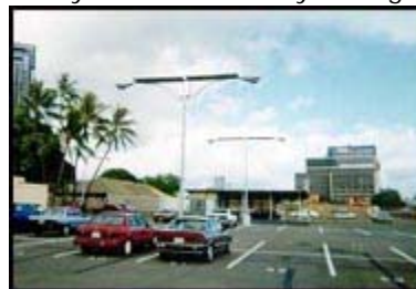
Solar lighting in the PJKK federal building parking lot
