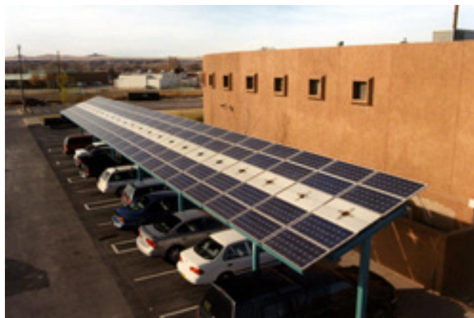
Figure 6-2: Parking Shade Mounded PV (photo credit – Sandia DOE/NREL)
