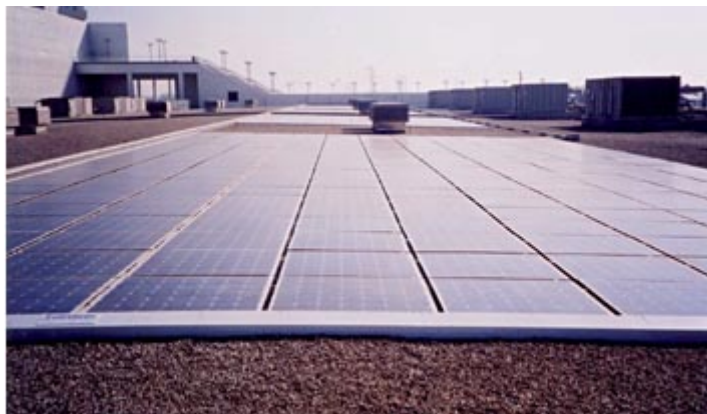
Figure 6-1: Flat Roof PV System (image courtesy PowerLight Corporation)
