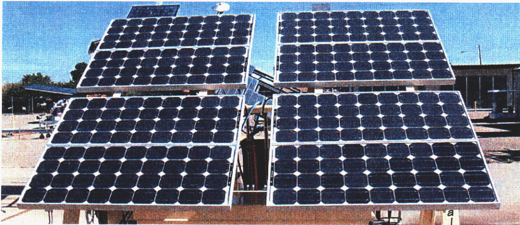
Figure 2. Photo of FireFly 600 photovoltaic array with eight BP Solar, BP275, 75-W crystalline silicon photovoltaic modules.
