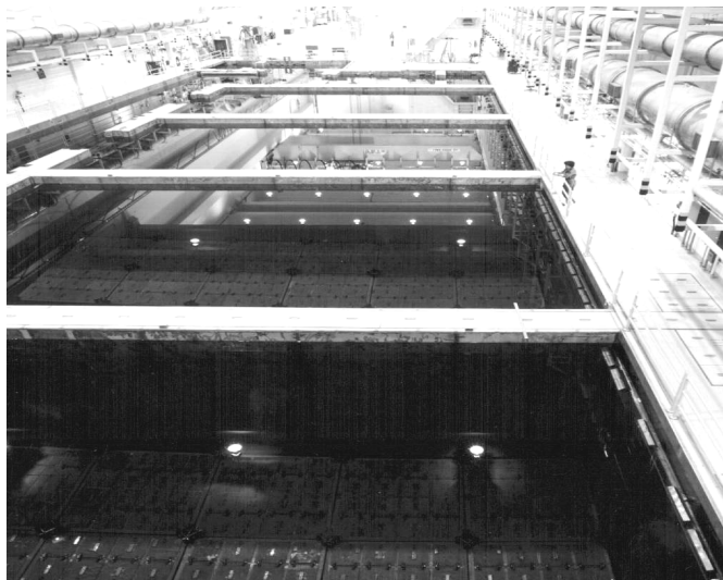
Figure 1. The modern steel-lined CP-666 Storage Pool at the Idaho Nuclear Technology and Engineering Center (INTEC)
