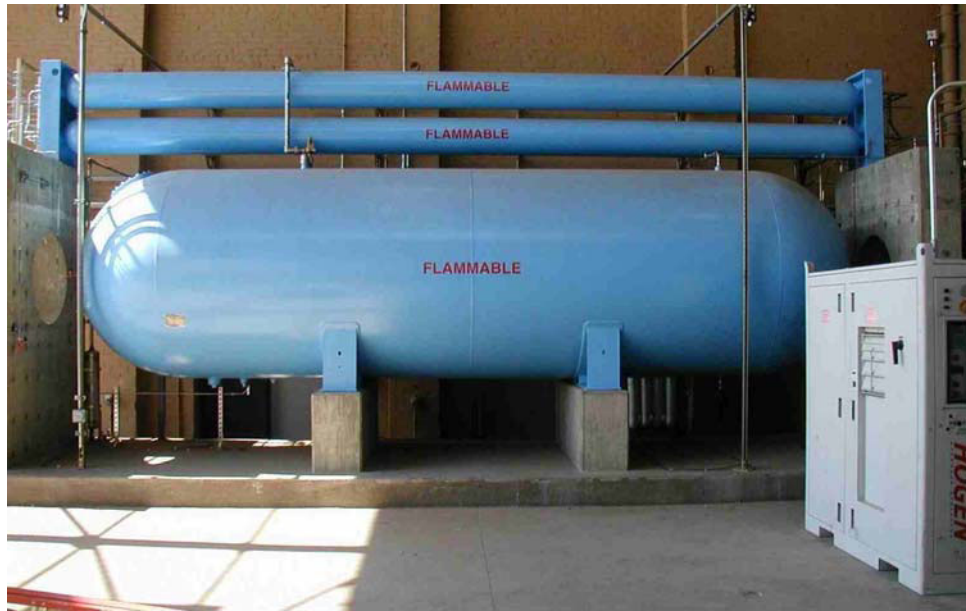
Figure 3. Low-pressure hydrogen storage tank (large, lower tank), high-pressure storage tanks (two upper tanks), and HOGEN fuel cell (right).
