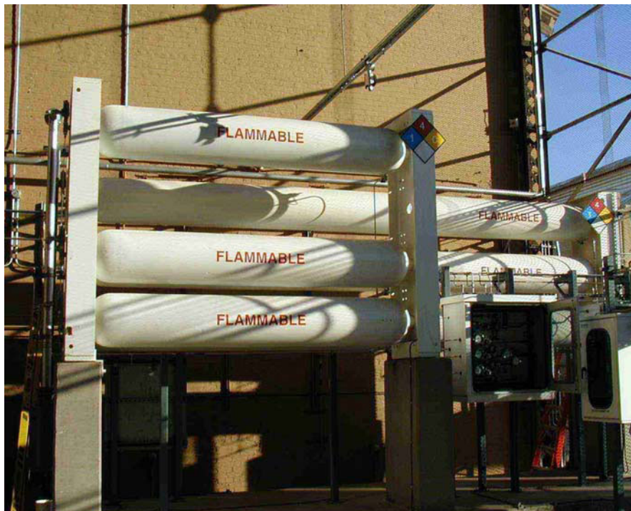
Figure 8. Compressed natural gas (CNG) tanks. In the near rack, the top tank is at high pressure; the two lower tanks are at medium pressure. The three low-pressure tanks are in the far rack.
