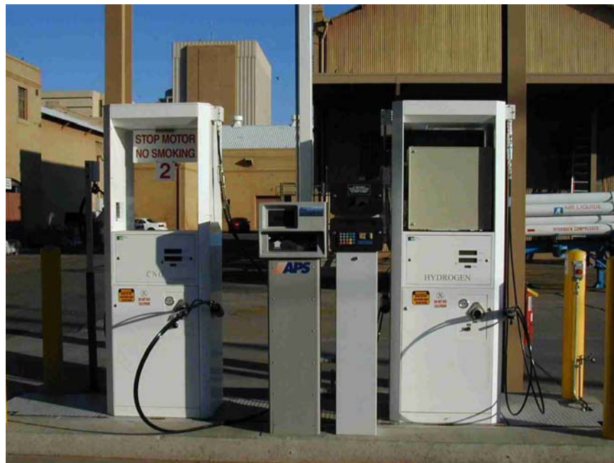
Figure 9. Compressed natural gas dispenser on the left and the hydrogen and hydrogen-blended fuels dispenser on the right, with the two credit card interface pedestals in between.
