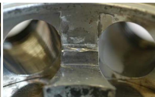
Figure 13. Wear on cut water near ports.
