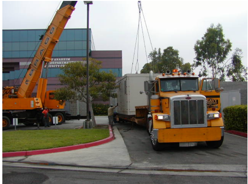
Image 17: Repositioning the fuel cell from the temporary site to the permanent position (May 21, 2004).
