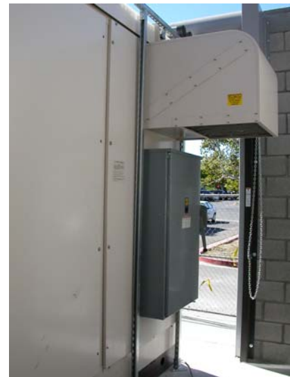
Image 23: AC disconnect on the fuel cell system (MD-1) is normally closed during normal operation.
