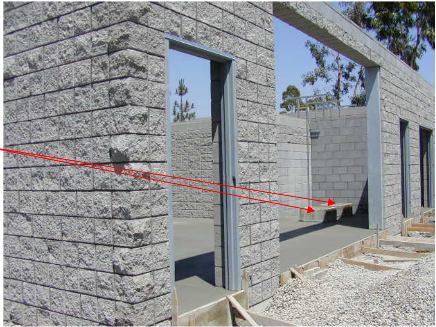
Image 15: Completed CMU wall and slab (August 2004). On the southwest wall there are two podium slabs for the new circulation pumps that were installed as part of the heat-recovery system. The pumps circulate some of the heat coming off of the fuel cell to heat the facility.
