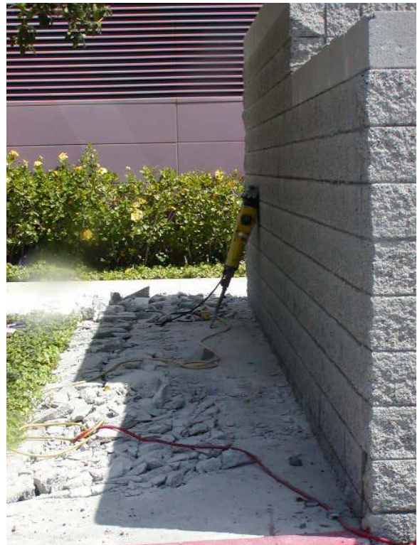
Image 8c: Demolition of original walkway adjacent to original CMU exterior wall (Project enclosed this CMU wall to install a new exterior wall).
