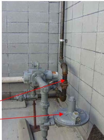
Image 27: The fuel cell system operates on a pressure rating of 10.16-35.56 cm (4-14 inches) water. The existing gas pressure into the facility was in the 10.16-22.86 cm (4-9 inches) water range with the boilers operating at 6 inches. As a result, the gas pressure needed to be increased and regulators were installed before the back-up boiler and before the fuel cell. This image shows the new service to the fuel cell and the new regulator.
