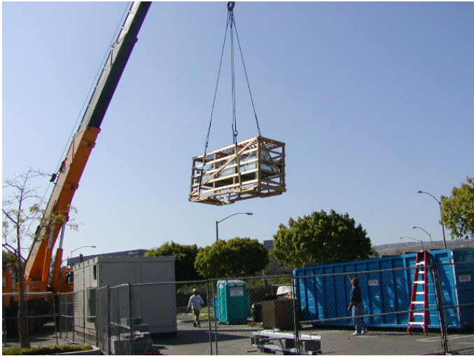
Image 12: Since the cooling tower would be mounted on newly constructed concrete slabs, it was also placed at the same temporary location as the fuel cell system until the concrete work was complete.
