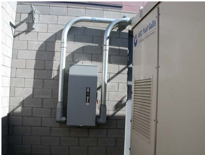
Image 22: AC disconnect outside the fuel cell system (normally open at MD-2) provides protection in case the system is switched to backup power
