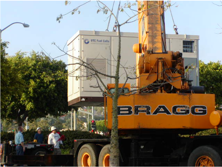
Image 11: Placing the fuel cell system required a crane to remove the plant from the truck and place it in a temporary location at the construction security site.
