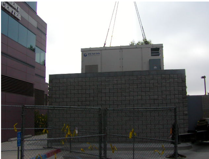
Image 18: Lifting the fuel cell over the CMU wall into its permanent enclosure.
