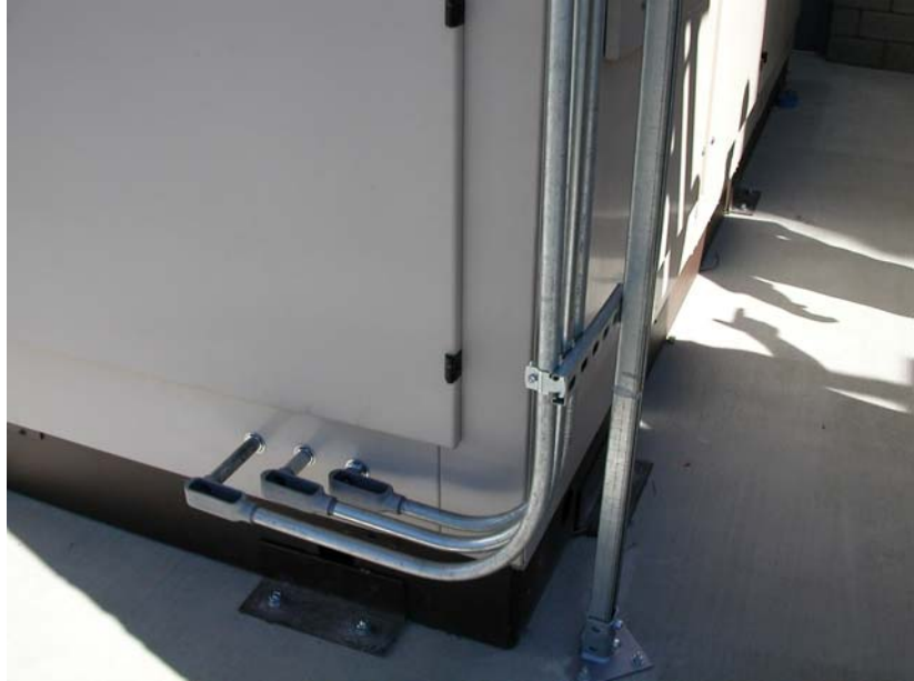
Image 21: 2.54 cm (1 inch) and 1.91 cm ( 3 / 4 inches) conduit for the phone wire, controls, and power to the cooling tower.
