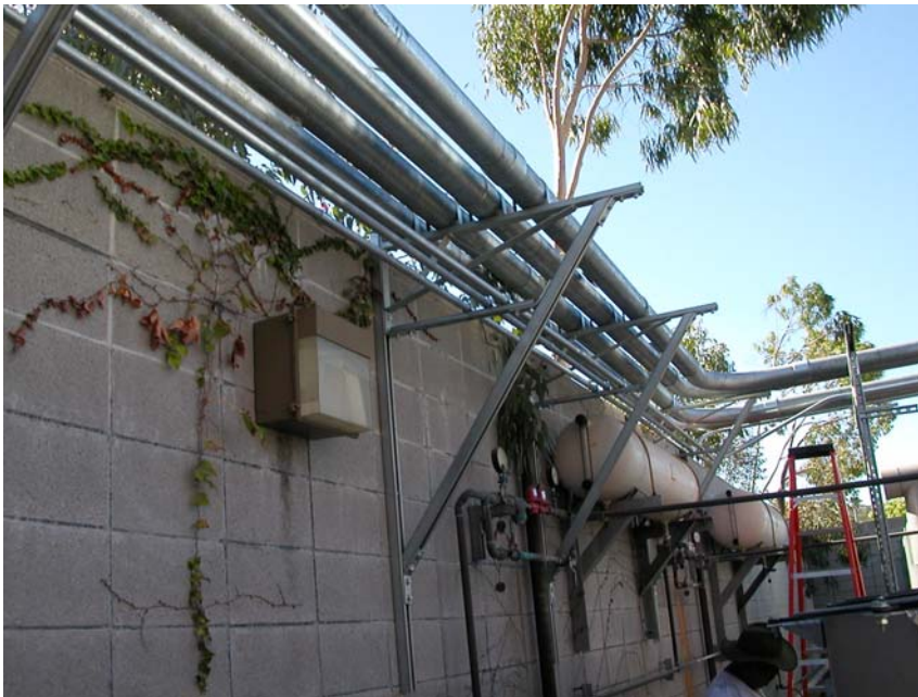
Image 20: Conduit uses a UniRack system to support the overhead installation.
