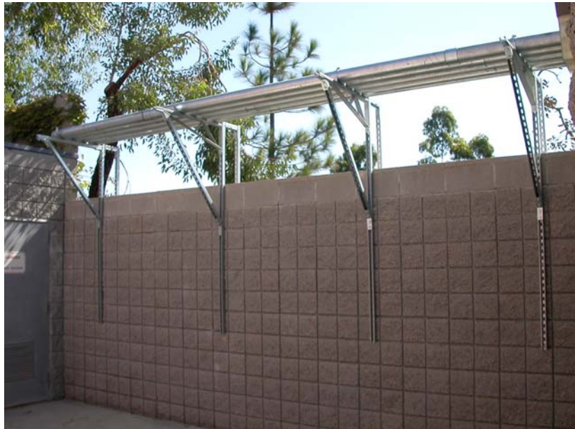
Image 19: All new conduit and piping associated with the Project was installed above-ground and mostly overhead. This photo shows the 10.16 cm (4 inches) power conduit, with protective relay conduit to the disconnect and the panel relay to the fuel cell 1.91 cm (3/4 inches), and conduits for telecomm and controls.
