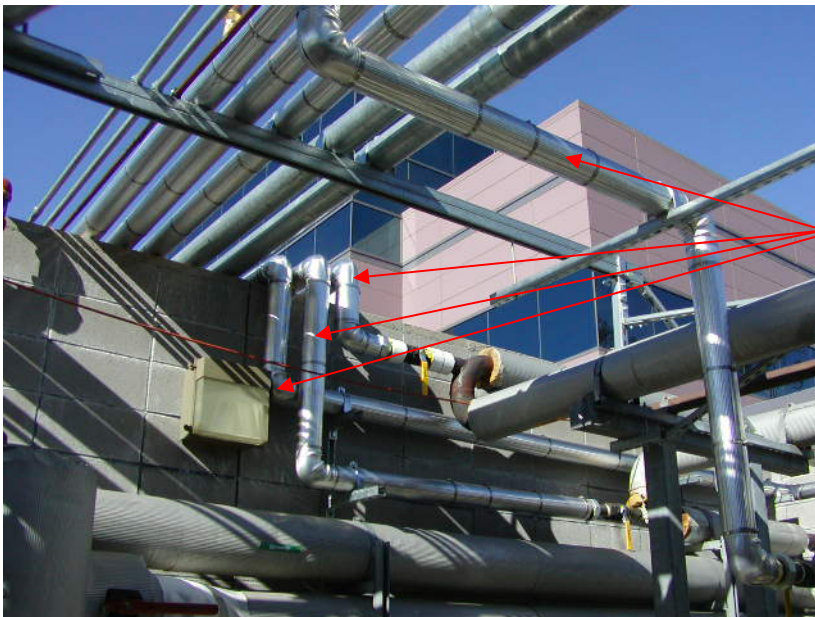
Image 30: The Hot Water Supply/Return lines intersect the original facility heating lines providing heat off of the fuel cell to the facility.
