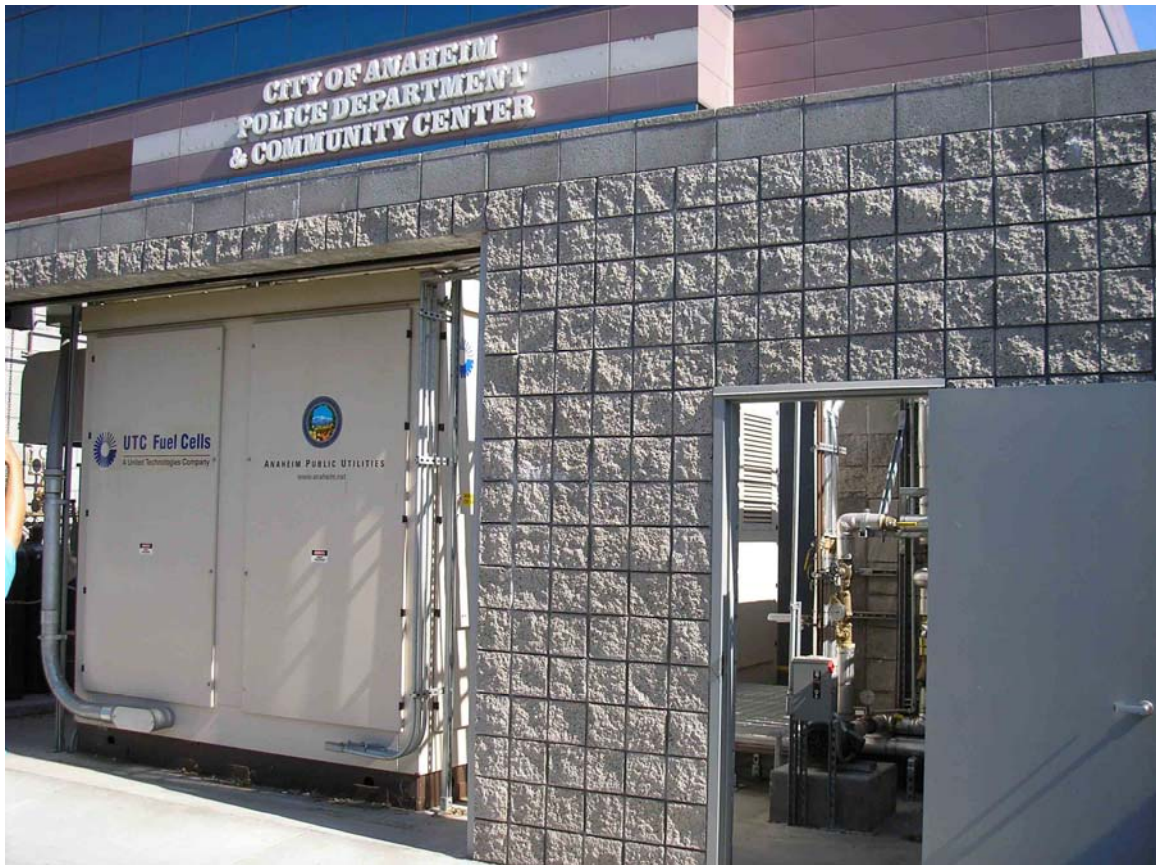
Image 31: Completed project shows the fuel cell to the left of the hot water return pumps. A roll-down door at the front of the fuel cell keeps the site secure. The fuel cell runs continuously at an average peak of 198 kW.
