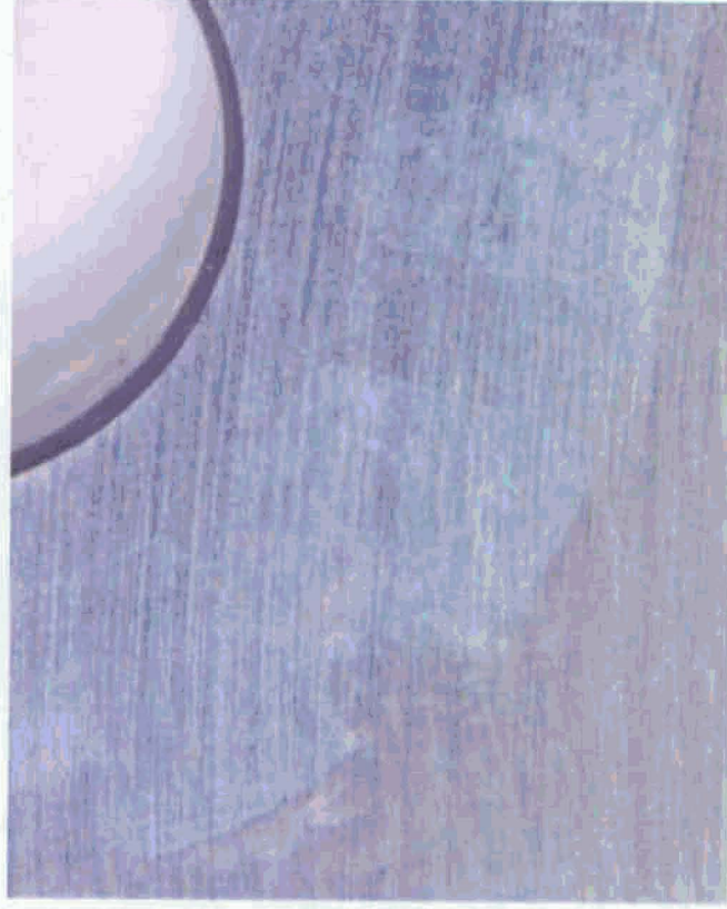
ASW KE0122 X 10 No Crevice Corrosion
