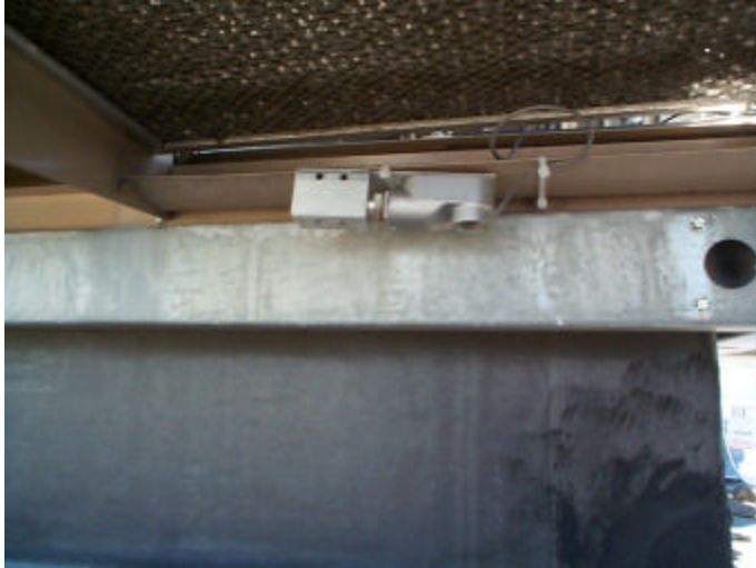
Figure 11. Ambient Temperature Sensor Under Fresh Air Intake
