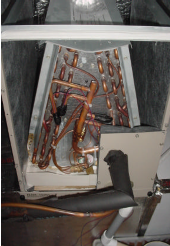
A-frame coil arrangement
