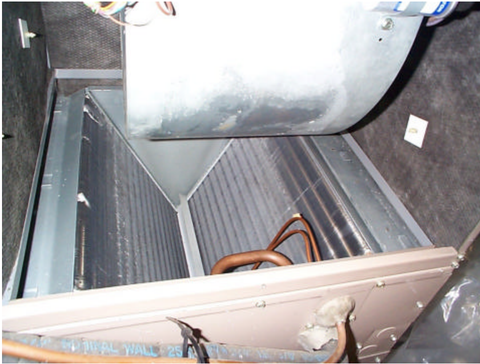
Figure 11. Coil in AHU #2
