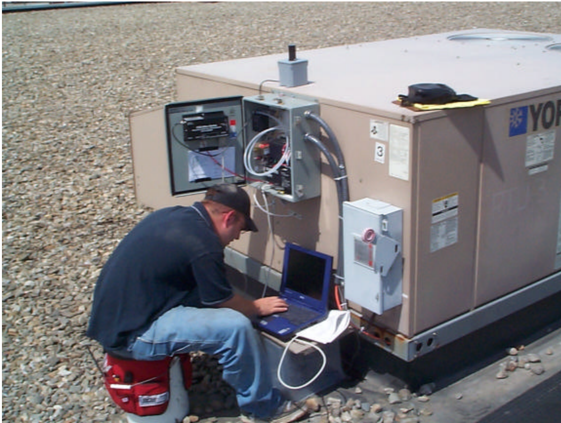
Figure 1. RTU With DAS System Installed
