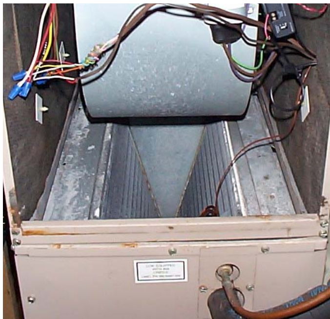
Figure 4-1. Residential Air Handler (Site 1, 2 nd Floor Unit)
