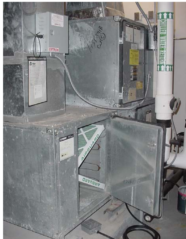
Figure 4-2. Commercial Air Handler (Site 7)
