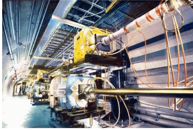
Figure 1 View of the PEP-II tunnel.
