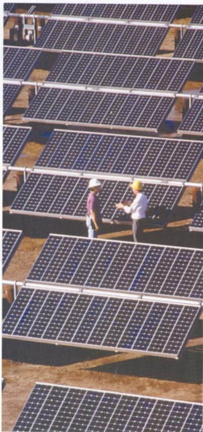
Photovoltaic technology (PV) uses solar panels to convert light from the sun to electricity. PV can be used nearly anywhere because normal daylight is all it takes for a solar system to operate effectively.
