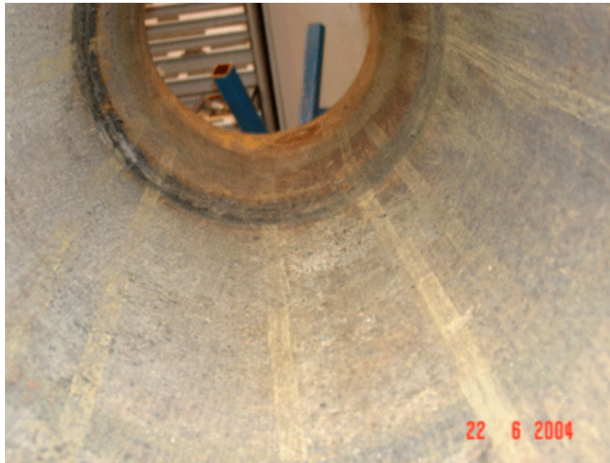
Figure 9. Cast-Iron Pipe ID after Cleaning
