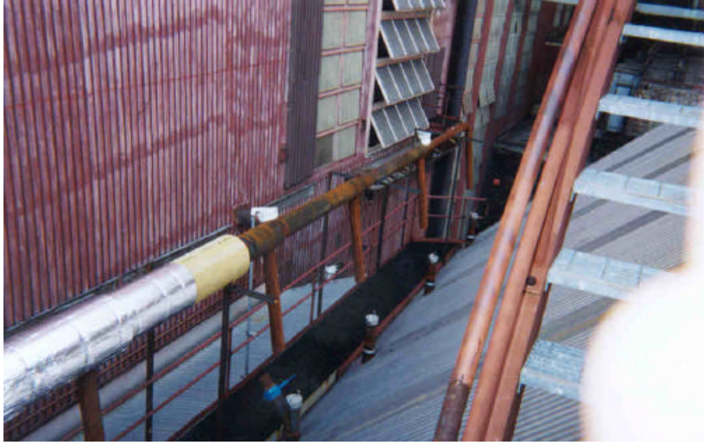
Figure 3.2-5 Slipstream Sample Rake Header at Main ESP Inlet Transition
