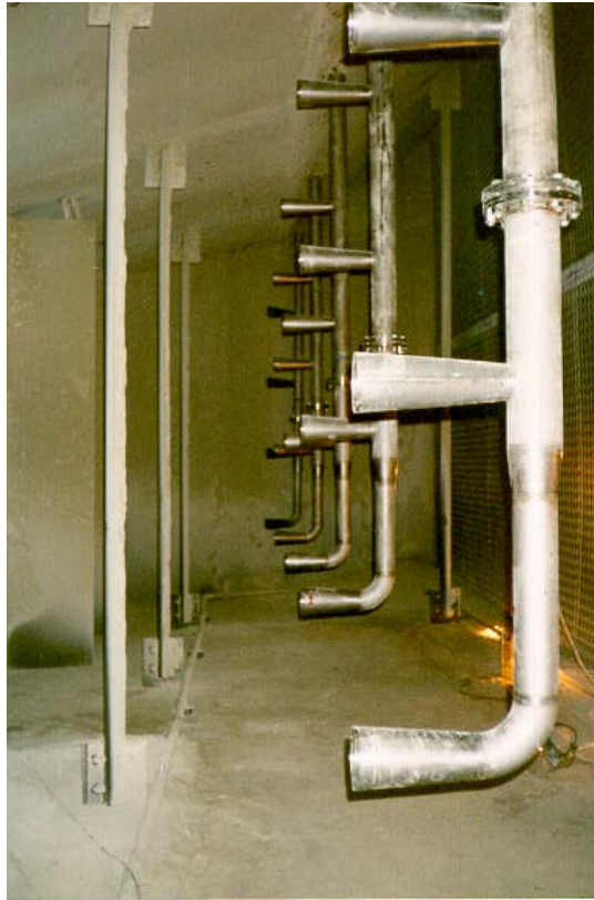
Figure 3.2-3 Slipstream Sample Rake Installation
