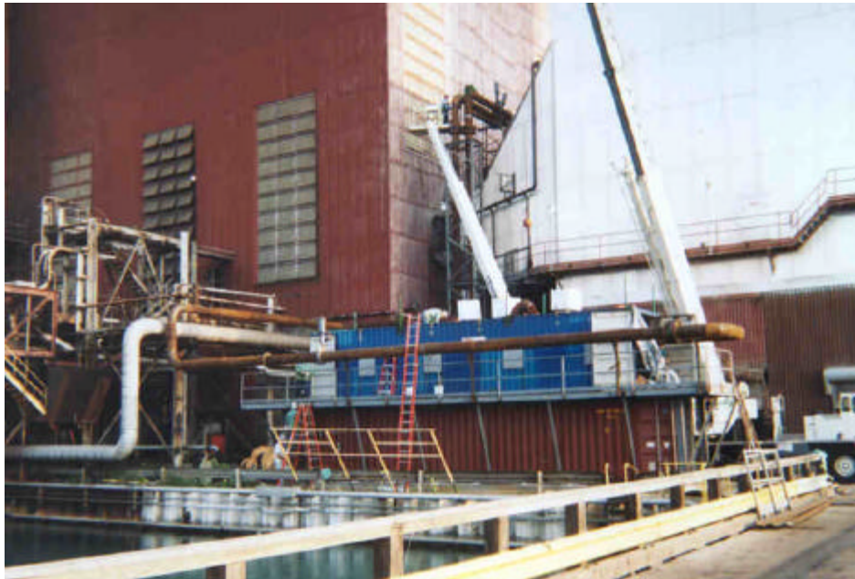
Figure 3.2-4 Pilot ESP Installation at Waukegan Unit No. 8
