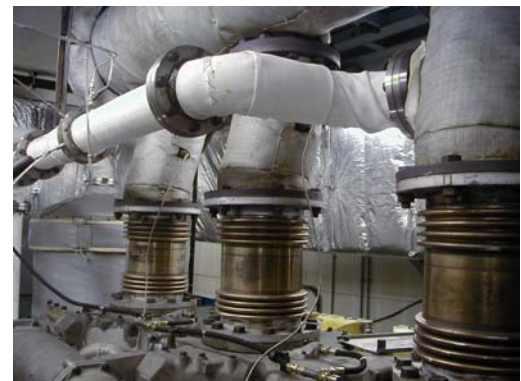
(c) The pipework from the exhaust to the non-thermal plasma system
