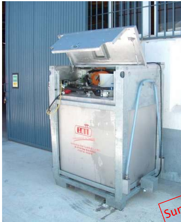
Figure 17: Urea Solution (AdBlue) Filling Station
