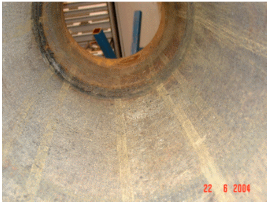
Figure 10. Cast Iron Pipe ID after Cleaning
