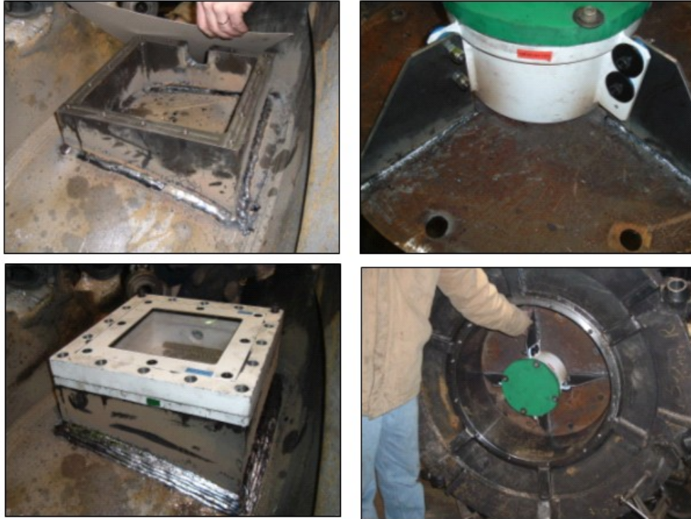
Figure 5.28. Installation of the HS-LW drum mounted component enclosures on a 7LS shearer drum. This tailgate drum, along with its companion headgate drum, was installed at the longwall of CONSOL's Robinson Run Mine.
