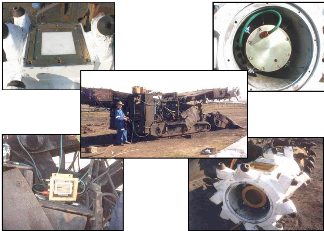
Figure 5.1. Installation of HS-3 on an HM-31 continuous miner at SASOL Fuel in May 2001
