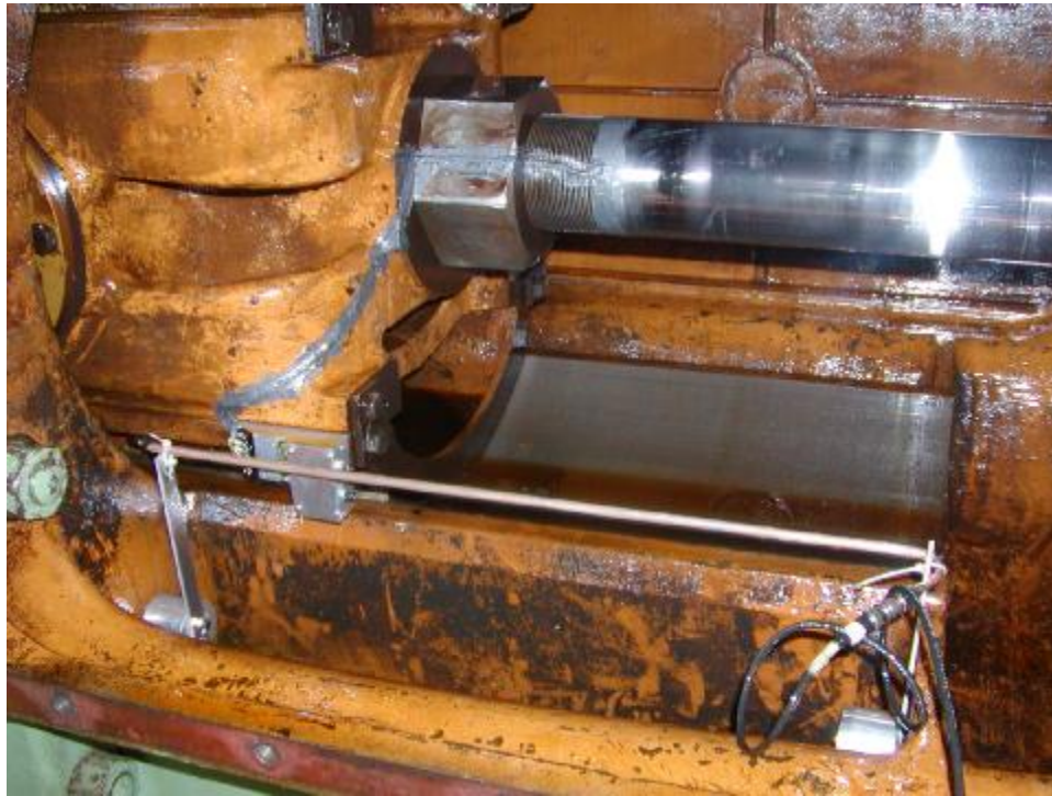
Figure 5. Rod Load Monitor Installation
