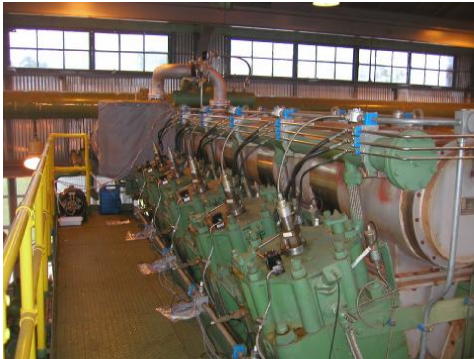
Figure 2. Power Cylinder, Left Bank
