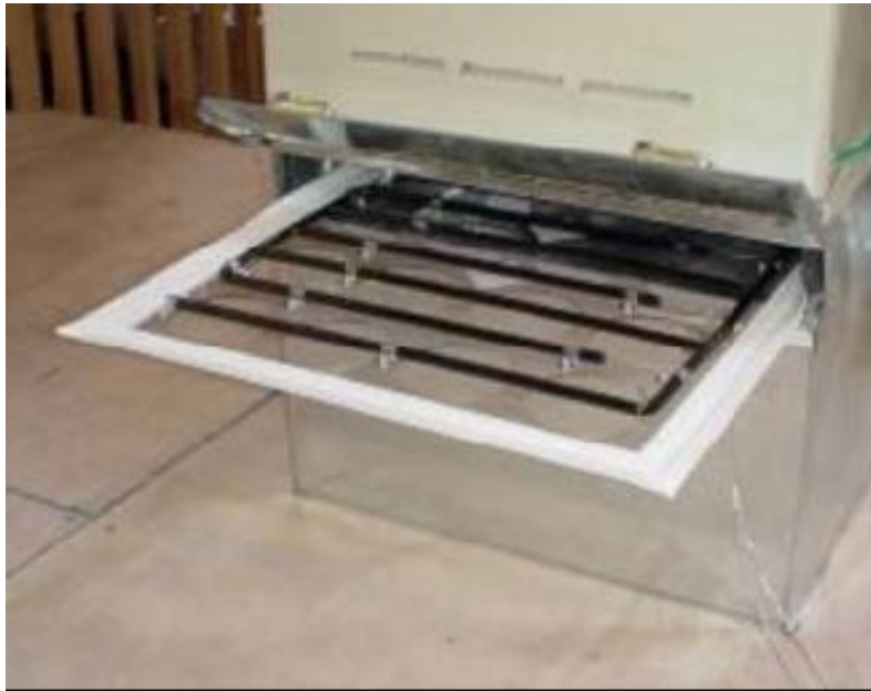
Pressure matching using an auxiliary fan and flowmeter Flow plate used to measure air handler flows (Paul Francisco, ECOTOPE, Inc.)
