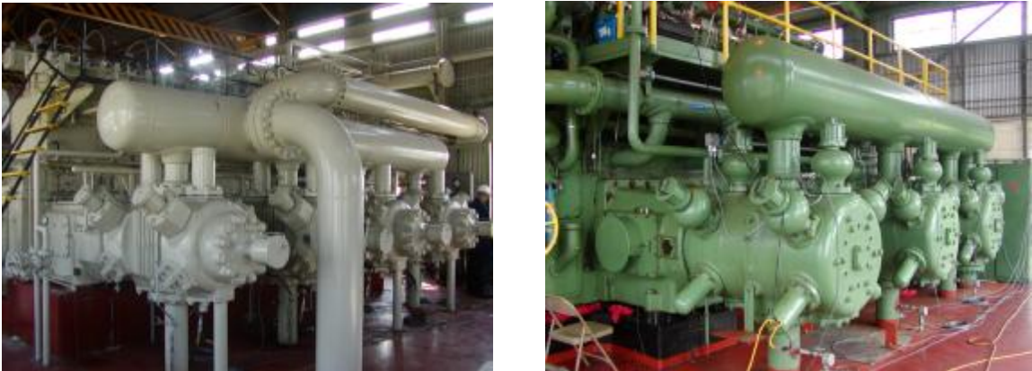
Figure 1. TLA6 (2000 HP) and GMW10 (2500 HP) in Pipeline Service
