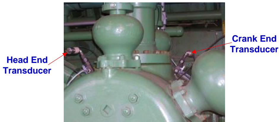
Figure 8. Compressor Cylinder and Pressure Transducers on each End
