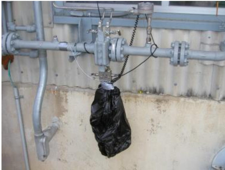
Figure 18. Flow Transmitter Connections to Orifice in Fuel Gas Line (GMW10, Williams Sour Lake Station)
