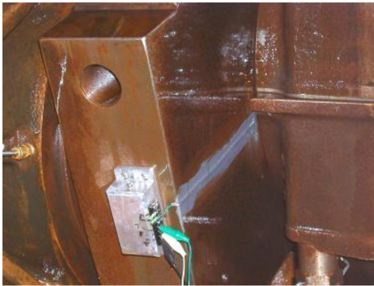
Figure 16. Strain Data Capture Module Installed (GMW10, Williams Sour Lake Station)
