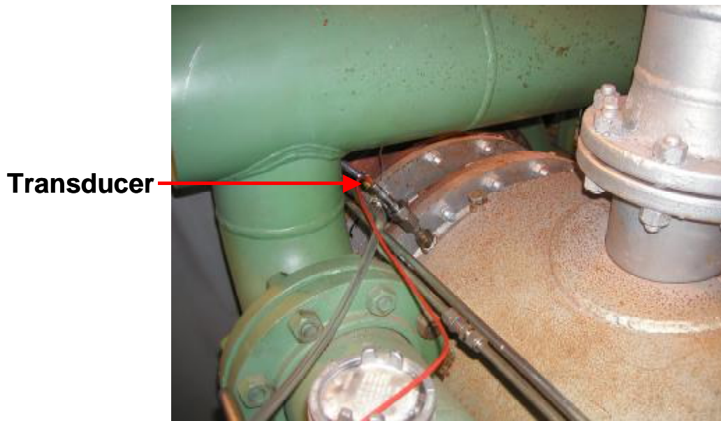
Figure 12. Pressure Transducer in Exhaust Manifold (GMW10, Williams Sour Lake Station)
