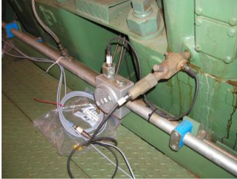
Figure 9. Details of Power Cylinder Pressure Transducer Installation
