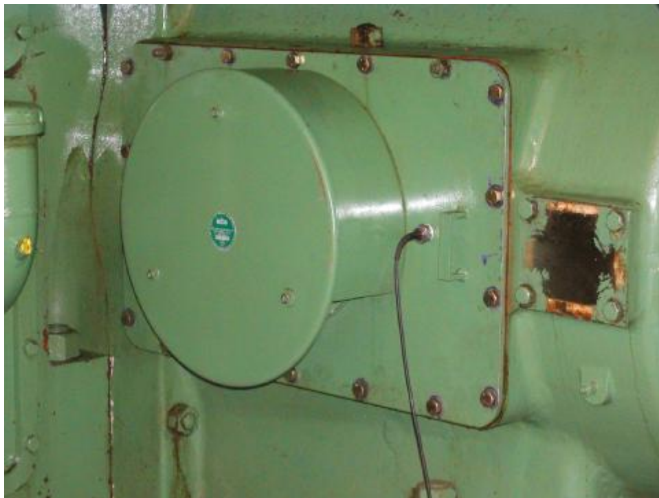
Figure 21. Cable from RLM Antenna (GMW10, Williams Sour Lake Station)
