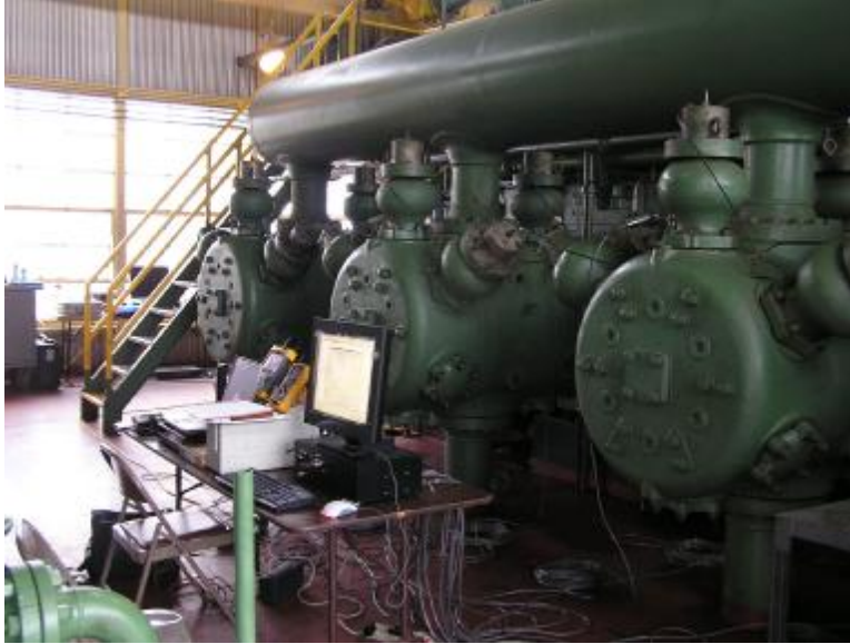
Figure 90. GMW10 Compressor Cylinders with Pressure Transducer Installed
