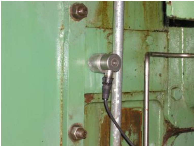
Figure 15. Accelerometer Mounted on Frame (GMW10, Williams Sour Lake Station)
