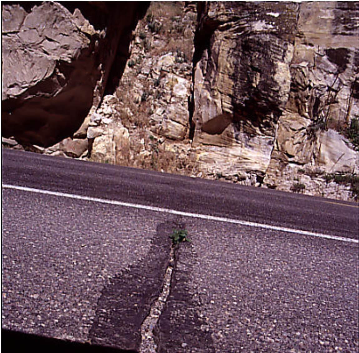
Figure 1-2. The first step to improved oil recovery is to admit that you have a fracture problem. Typified by this photograph of a crack in the pavement opposite an outcrop of Tensleep Sandstone in the Wind River Canyon, engineers sometimes try to “pave over” fractures and hope that the problems will go away. However, as the photograph above shows, the fracture opens up each Spring no matter how much “paving over” takes place. The fracture in the pavement actually is part of a very large (over 40 m high) fracture that is obvious in the vertical outcrop. There is little hope that putting tar into the fracture each summer will ever stop fluids from moving through the large fracture and disrupting the pavement.
