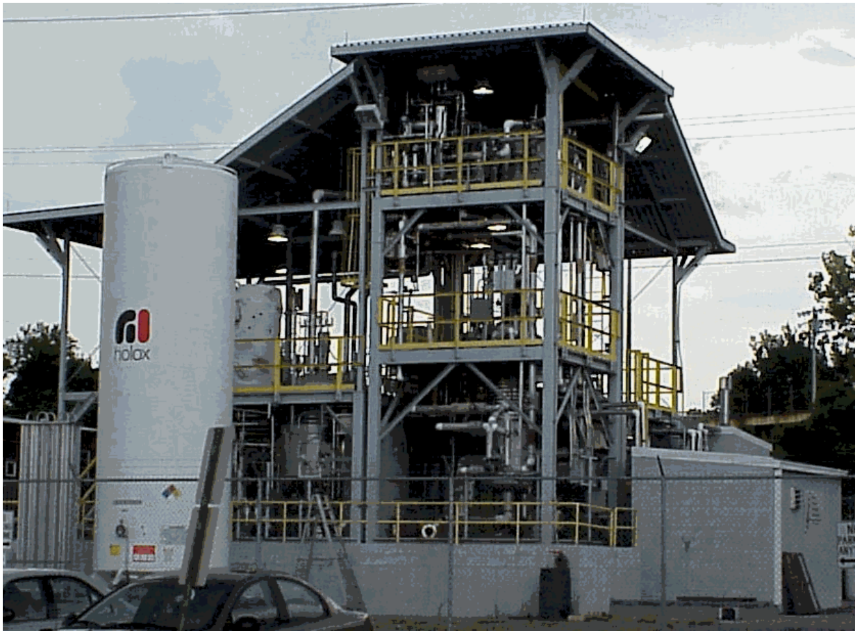
Figure 1. Filtration Research Engineering Demonstration
