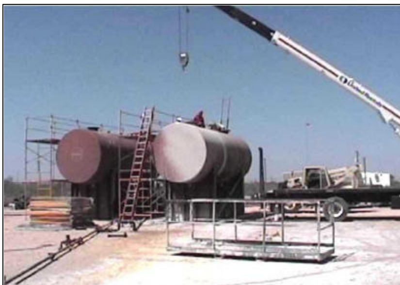
Figure 1. View of horizontal tanks used for 1999 field demonstration.
