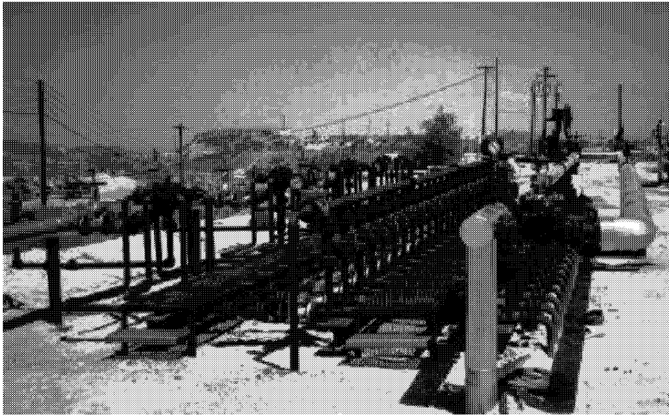
Figure 6-4: Auto well tester #1 unit for metering Pru Fee producers on-site. The unit was installed by Aera Energy in preparation for beginning steam flood of "300-series wells in early 2000.
