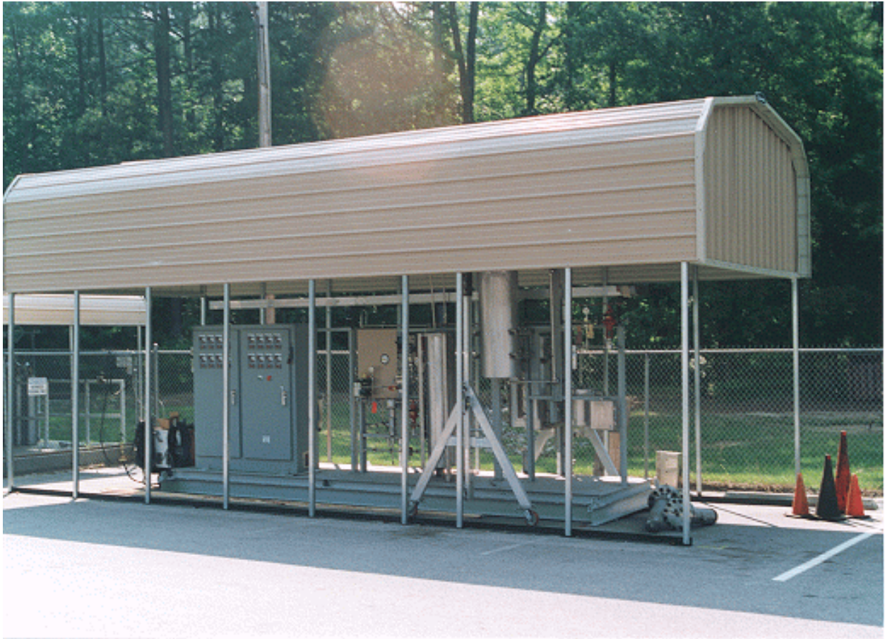
Figure 1. The weather-protection canopy has been installed over the enlarged Skid-Mounted DSRP unit while it is at RTI undergoing final fabrication. This same canopy will be used during the field test at PSDF.
