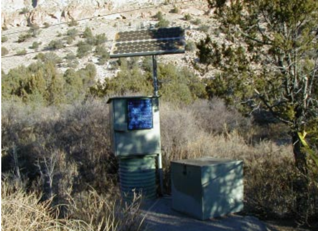
Figure 15. Automated Storm Water Station E042 LA Canyon Near LA
