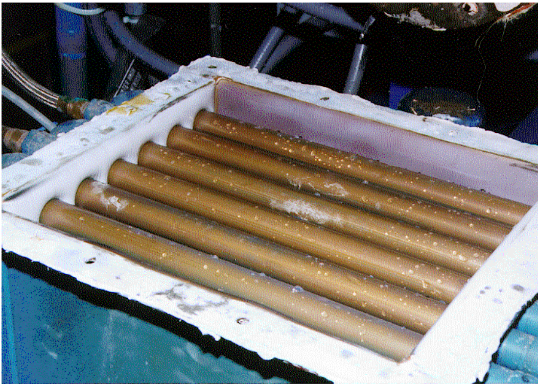
Figure 5.3 Top of CHX ® Heat Exchanger After Washing
