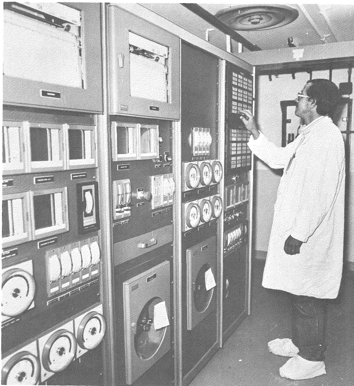
FIGURE 27. Process Control Instrument Panel in RADTU Facility.
