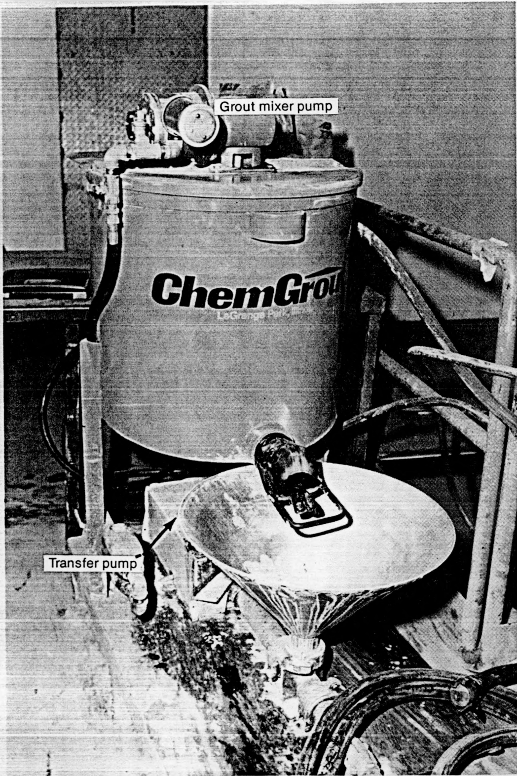
Figure 2. WEDF solidification grout mixer and grout transfer pump.
