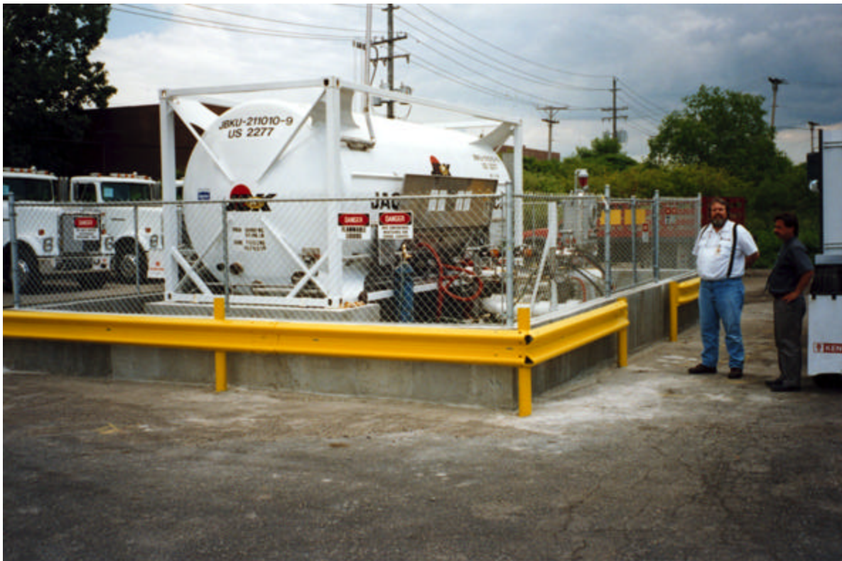
Figure 6. Temporary Fueling Station at TDM
