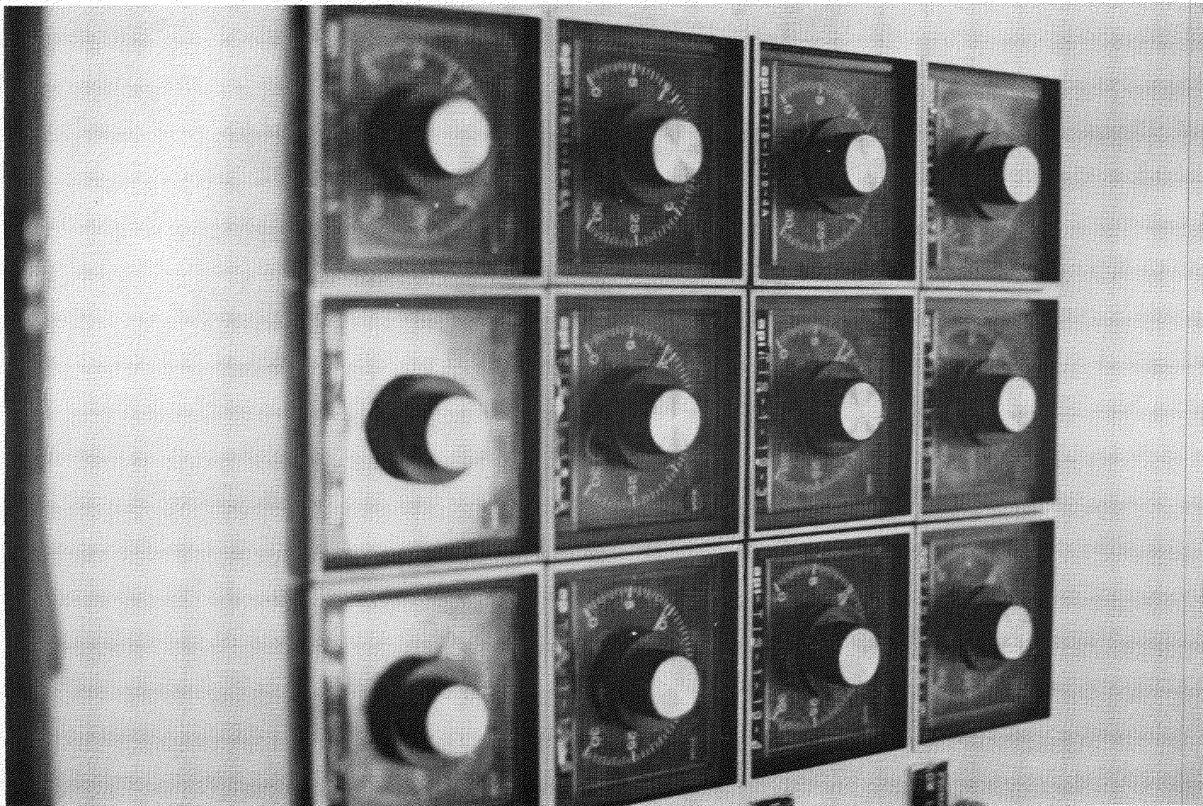
Figure 37. Pump bearing temperature indicators. (Forward canting of these meters would improve their visibility.)
