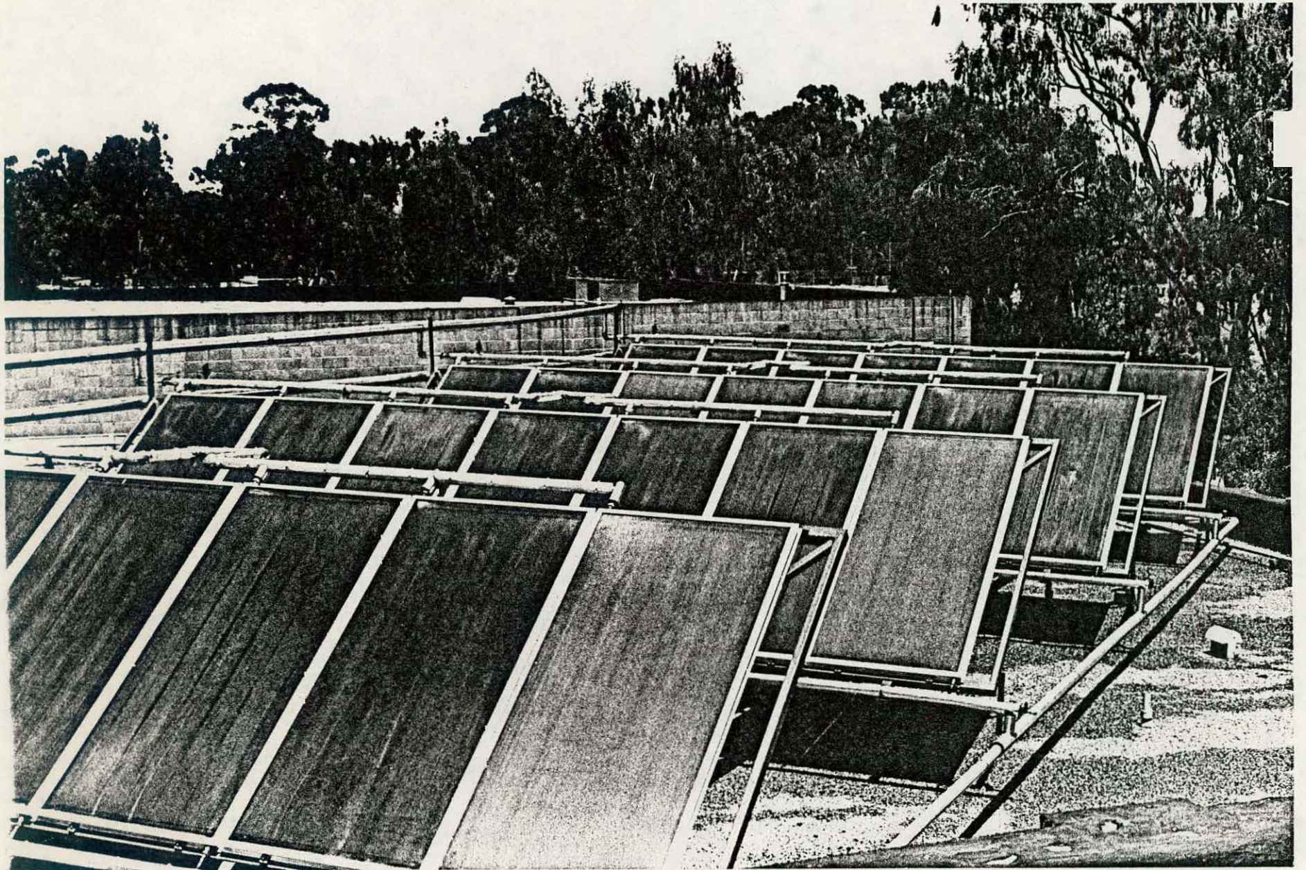
Four banks of solar collectors.
