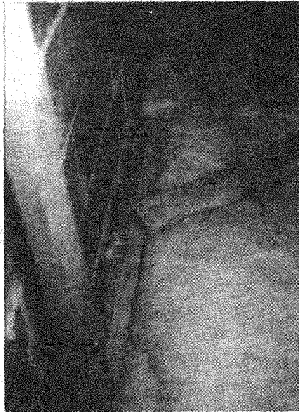
GAPS AT ATTIC FLOOR
