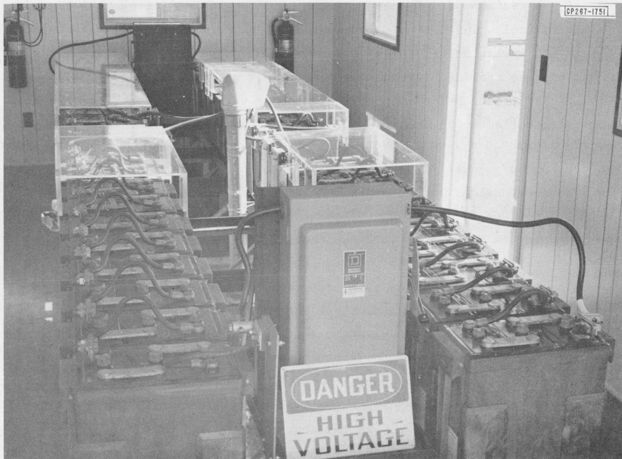
Fig. III-10. Interior view of the battery trailer.
