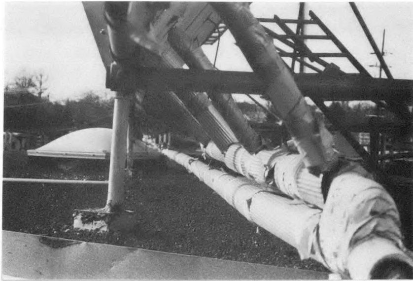
Figure C.19 Piping Located Close to Roof Surface
