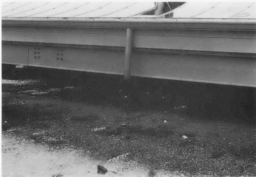
Figure C.3 Ponded Water on Roof Surface Extending Under Large Wooden Platform Supporting Solar Reflectors
