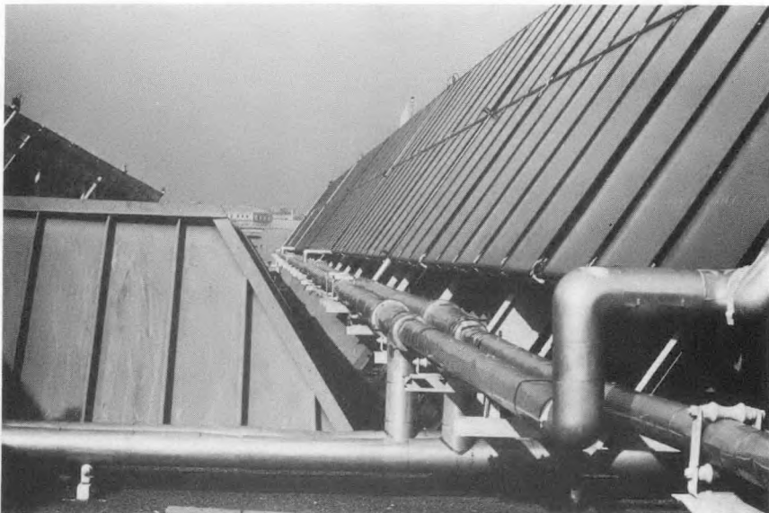
Figure C.20 Inadequate Clearance Between Front of Collector Array and a Mansard Style Roof Projection
