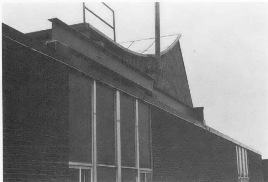
Figure C.6 Large Wooden Reflector Frame Supported by Exterior Walls and Columns of the Building
