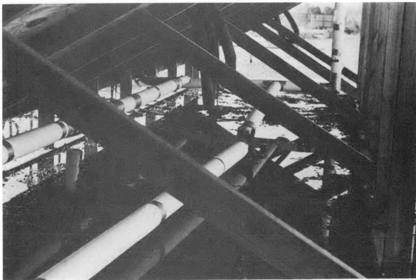
Figure C.18 Inadequate Clearance Between Wooden Collector Frames and Roofing
