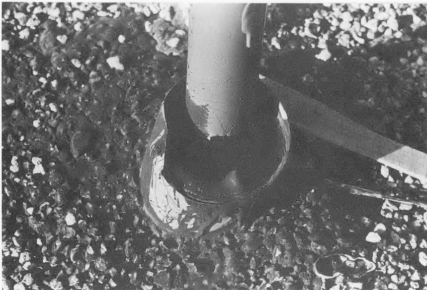
Figure C.10 Collector Support Column in a Tilted Pitch Pocket
