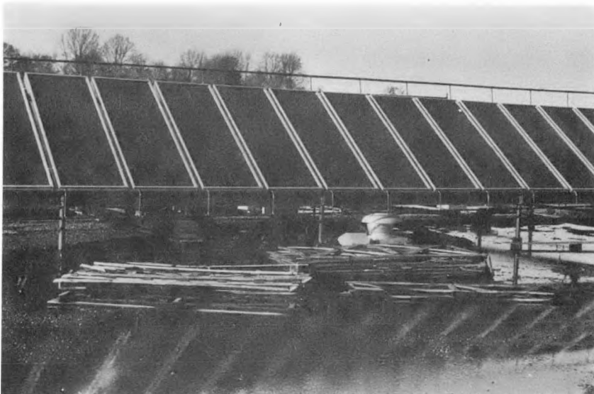
Figure C.34 Debris On Roof from Solar Installation
