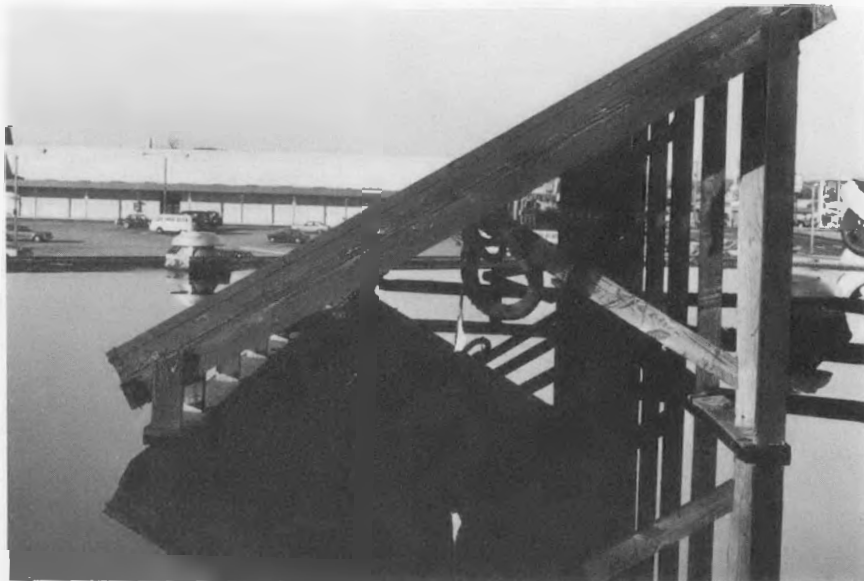
Figure C.12 Ponded Water Above the Bottom Surface of the Wooden Sleepers
