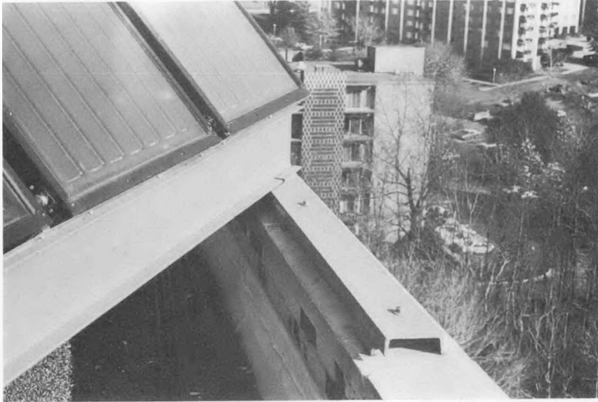
Figure C.9 Attachment of Collector Support Beam Using a Steel Clip Welded to a Channel which is Bolted to a Parapet Wall
