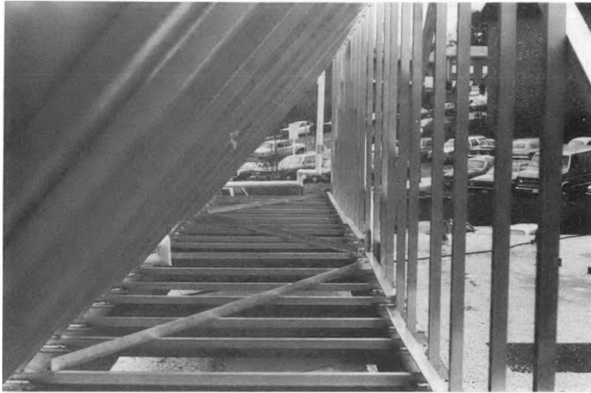
Figure C.17 Inadequate Clearance Between Steel Collector Frames and Roofing
