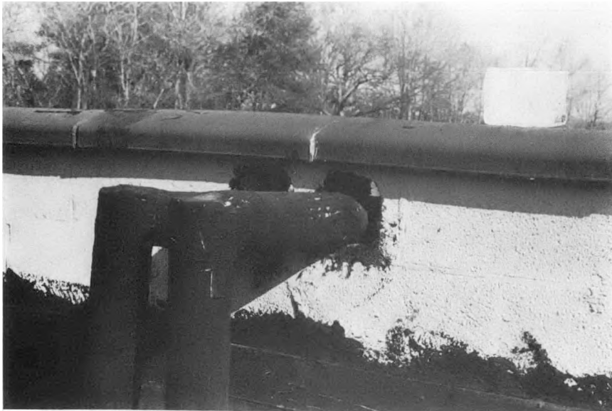
Figure C.29 Fire Wall Penetrated by Solar Piping
