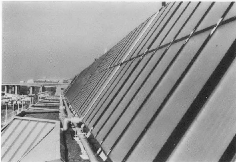
Figure C.27 Collector Array Installed Near Roof Edge
